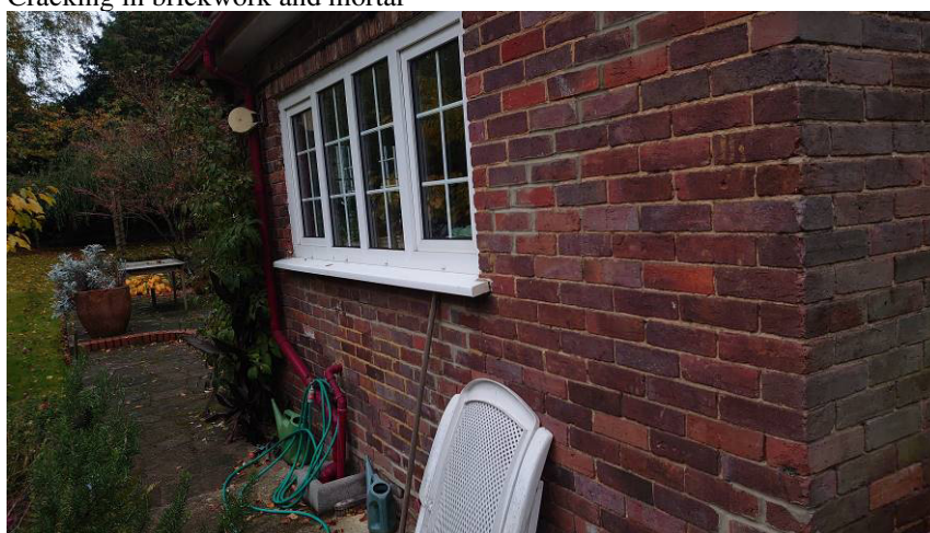
Previous repairs showing signs of opening up
