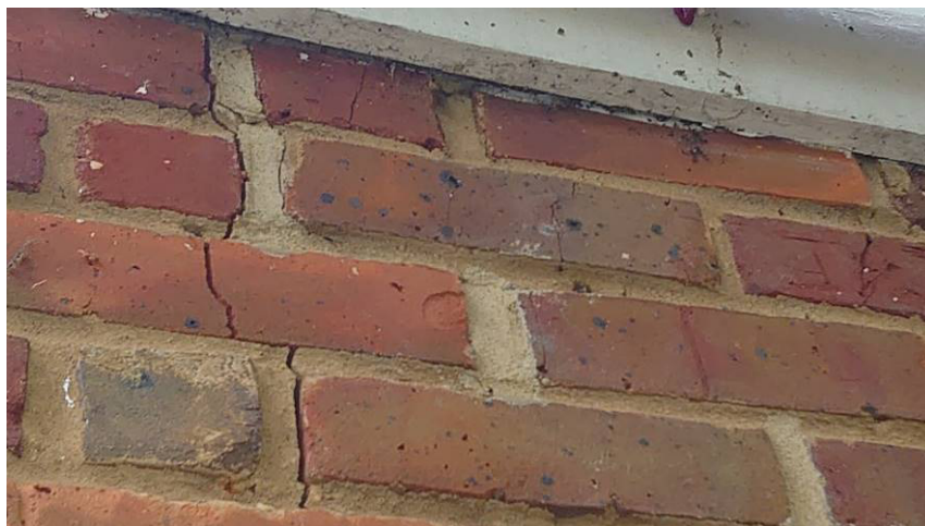
Cracking in brickwork and mortar
