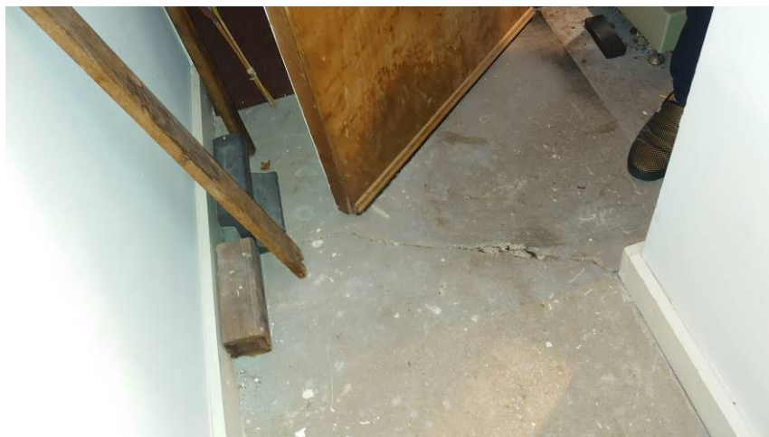
Cracking in ground floor
