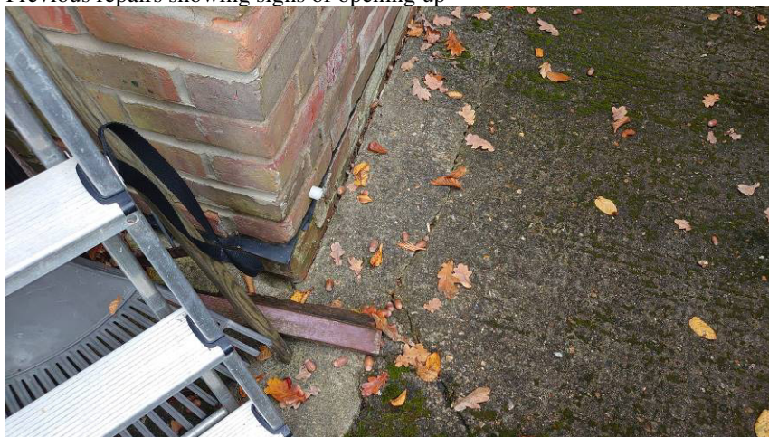
Settlement of wall below dpc
