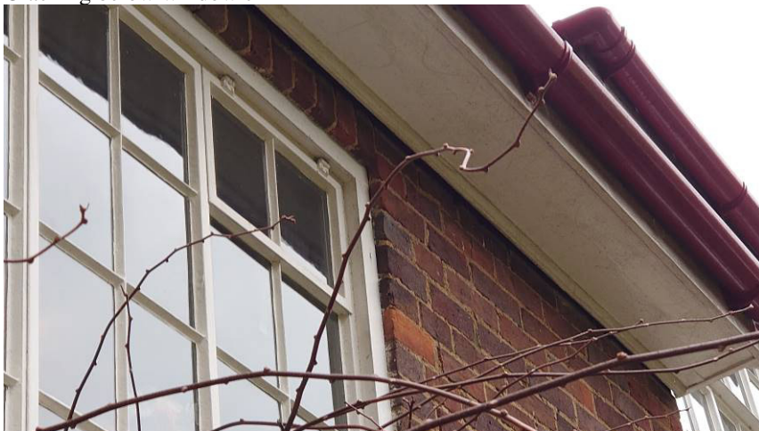
Gap at roof eaves and soffit due to outward movement of the roof
