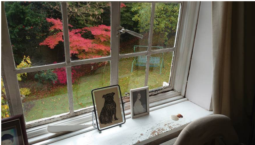
Outward movement of wall
