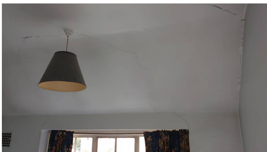
More internal cracks
