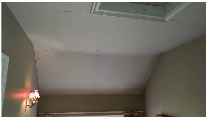
More internal cracks
