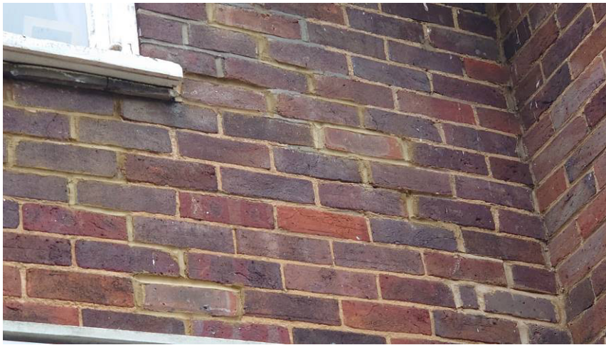
Cracking below window cill
