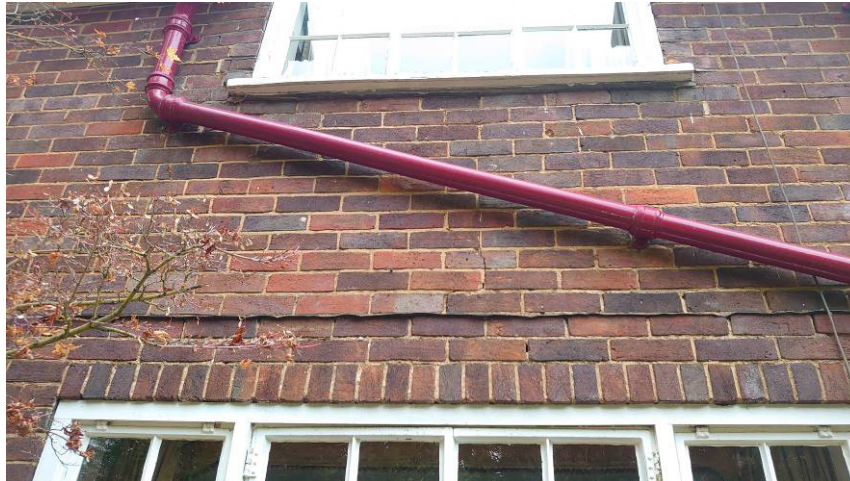
Outward movement of the wall
