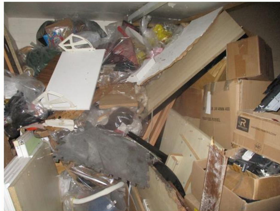
Photo No.22: Heaps of refuse, debris, materials and equipment noted inside toilet enclosure of units No.18/19
