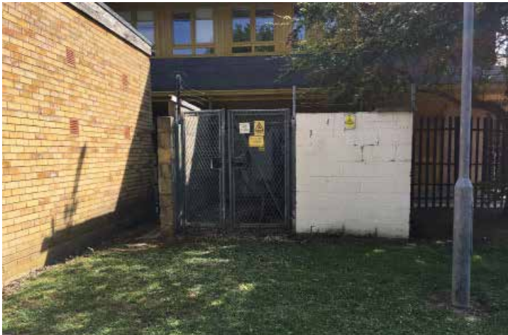
Electrical Sub Station
