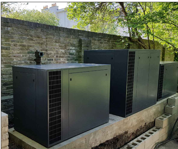
Typical A/C Unit Enclosure_ T4-1200 Acoustic Enclosure
