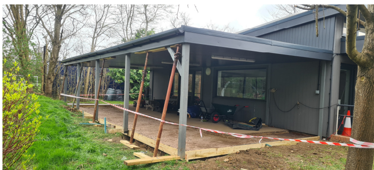
Images showing new roof and timber supports, and new floor before finish. March 2026.
