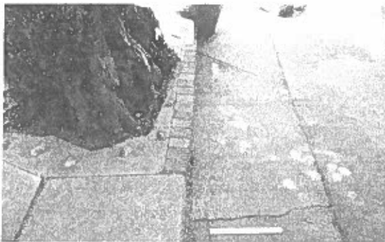
Figure 3 Crack in lifted garden path.
