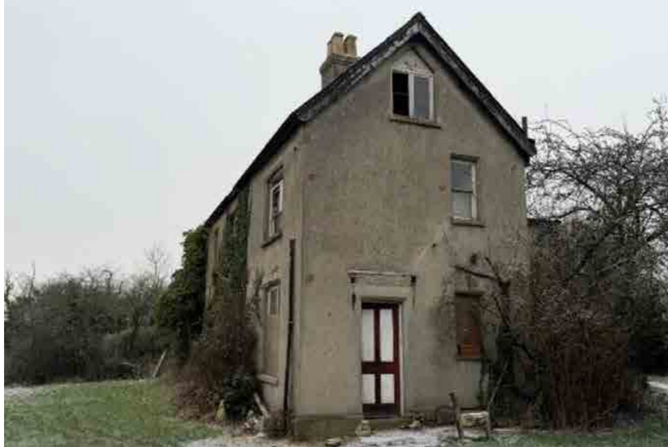
View of East Elevation of the farmhouse with repair work completed to the ground floor. Due to the presence of bats the repair work has been confined to that which is permissible under ecology constraints. Please see appendix for ecologist's letter to this effect.
