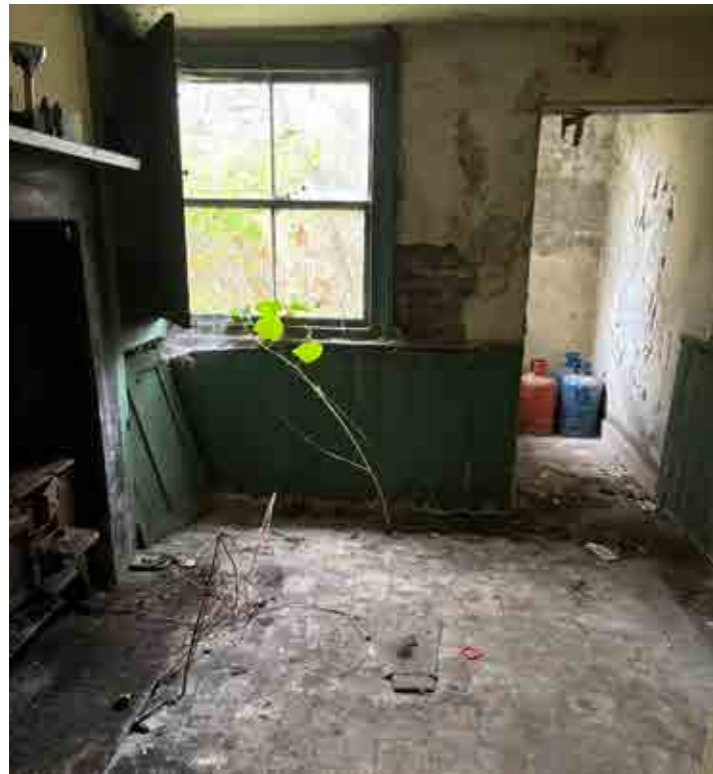
Existing view of the interior of the farmhouse showing Japanese knotweed growing up through the substructure. Please see appendix for report of Knotweed treatment completed to date
