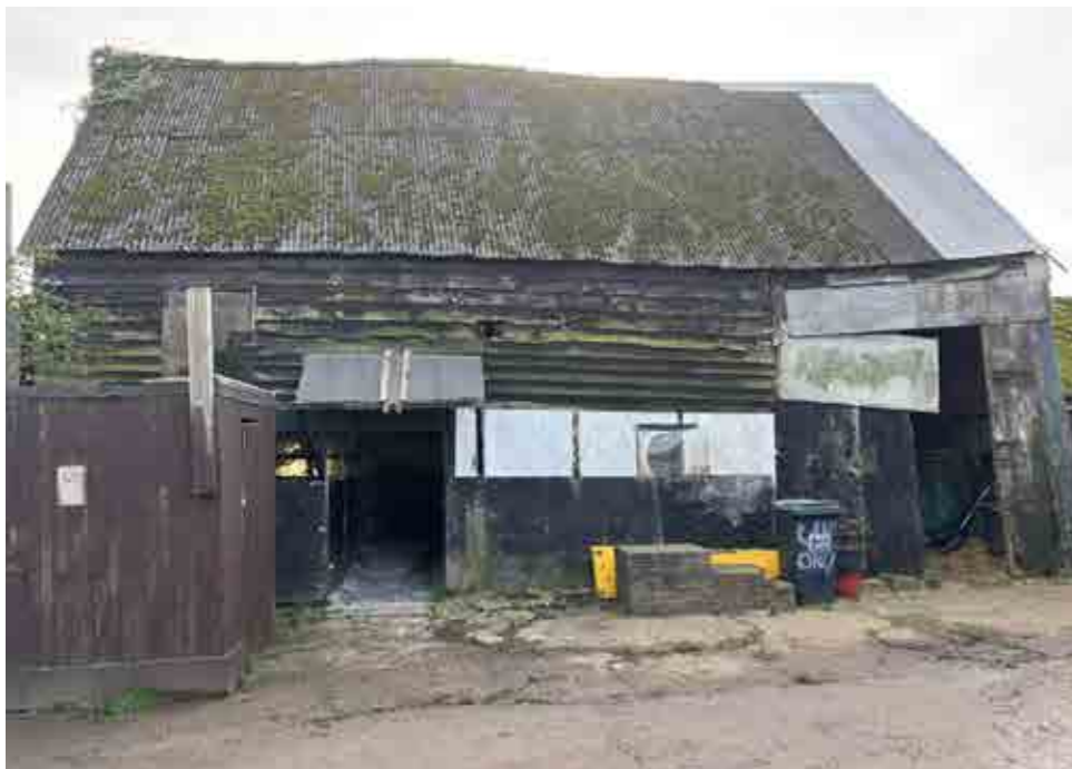
Photograph of the front of the existing retained heritage barn showing existing ground level sloping up to a raised internal floor level. The ground level in front of the barn will be reduced in addition to the internal floor level of the barn itself to align.
