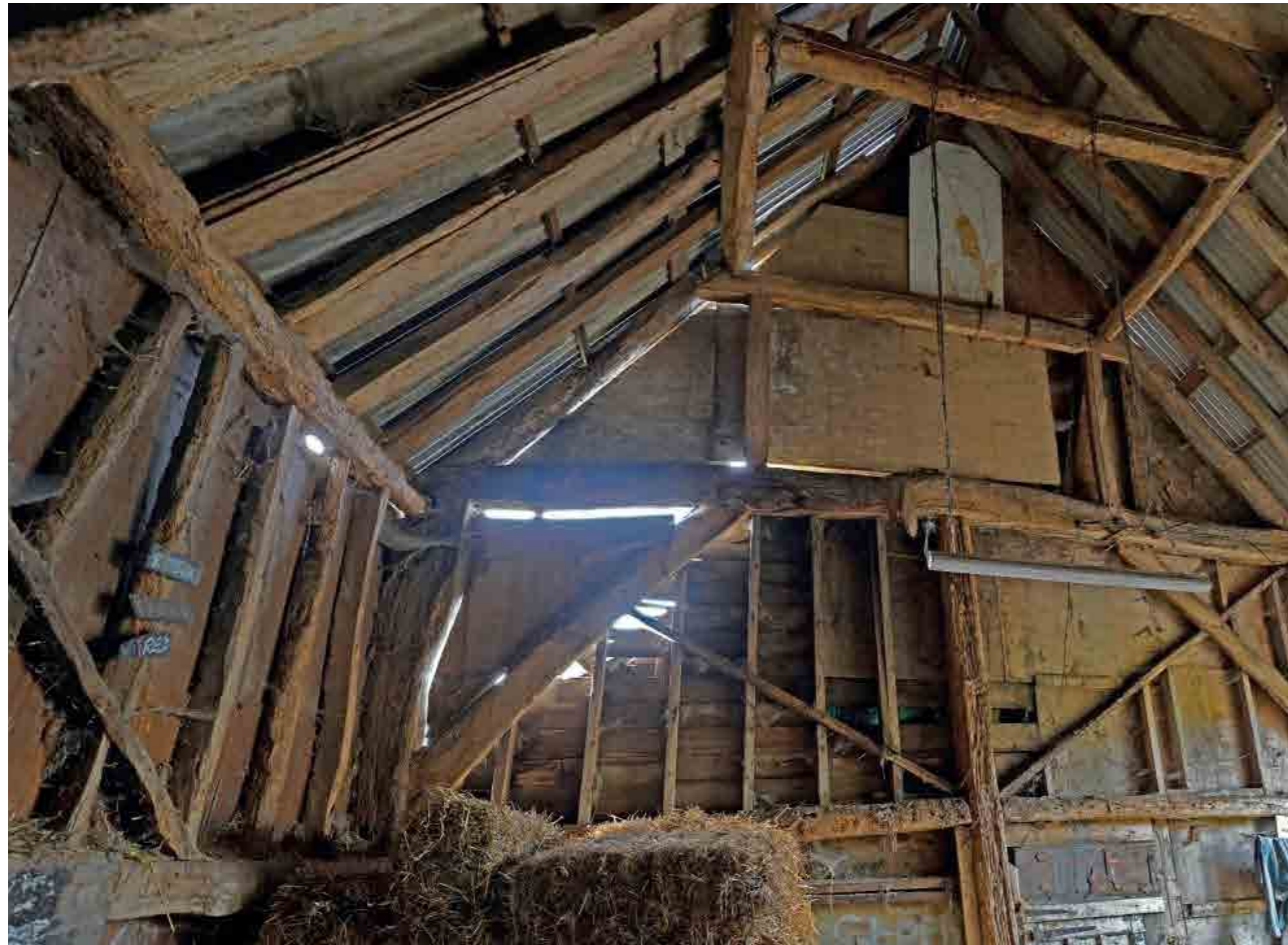
Internal view of the retained timber barn. The frame will be refurbished as part of the works so the barn can form the center of the customer arrival space. The incorporation of this structure at the heart of the scheme has inspired us to consider how the principle of solid oak framed-structure could be carried through the proposed building in a contemporary manner.
