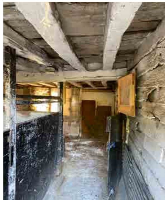
Photograph of the underside of the existing barn mezzanine. The existing height from floor level to underside of central beam is 1880mm at its lowest point requiring some reduction in floor level in order to make use of the barn feasible
