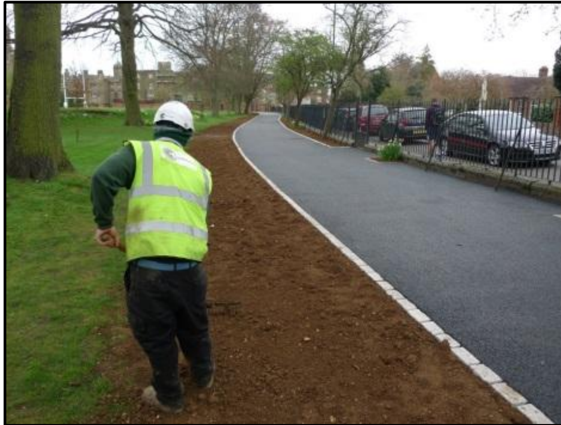
Fig 14 – All 'making good' topsoil will be BS3882 compliant and raked out by hand to no greater depth than 100mm.
