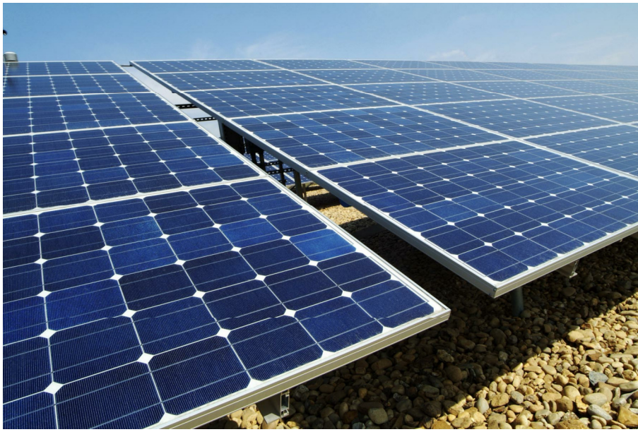
⑪ PV panels
