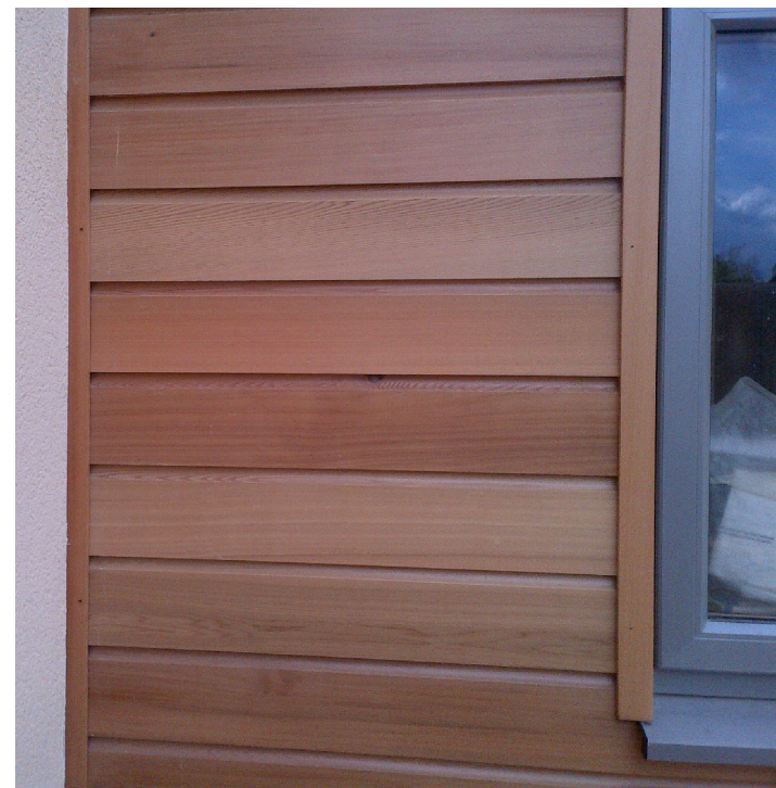
4 Timber Cladding British Red Cedar
