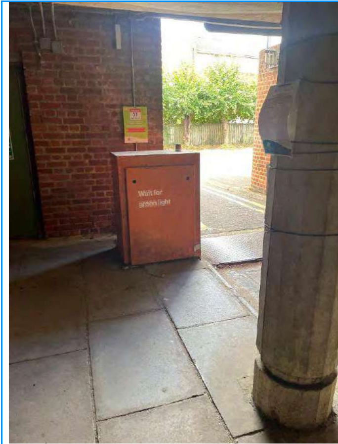
Electric box at carpark entrance
