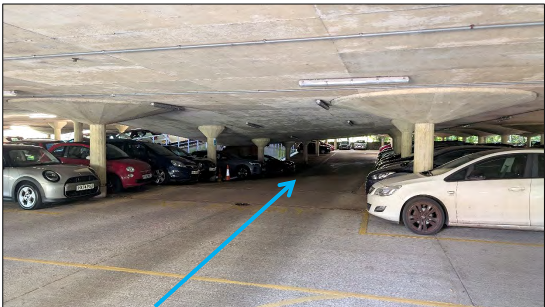
Photo 3 Interior of car park, showing depression in centre of car park
