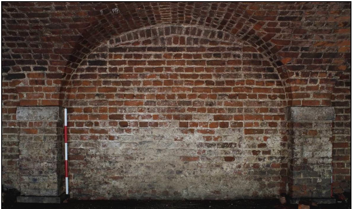
Plate 10: Blocked Opening to Room 9
