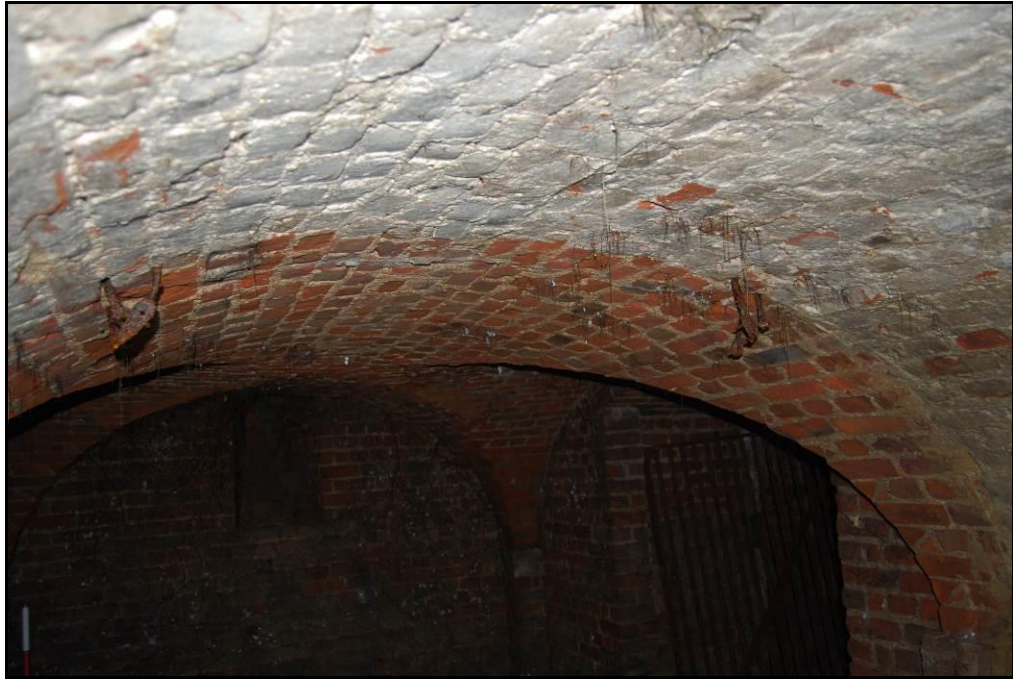
Plate 28: Nails in arch at west of Room 7
