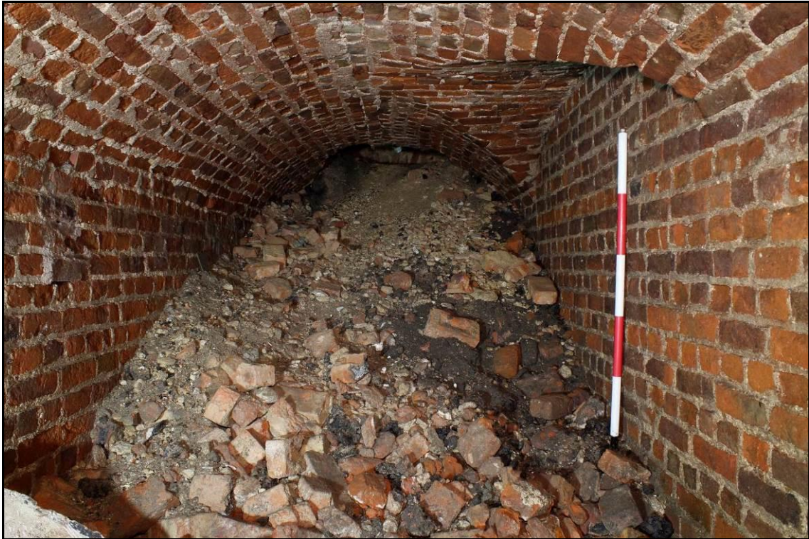
Plate 11: Rubble within Room 9, Looking South
