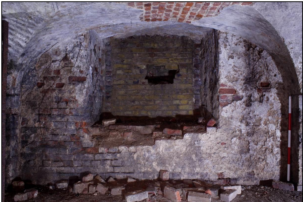
Plate 20: Blocked window, Lightwell beyond in Room 2
