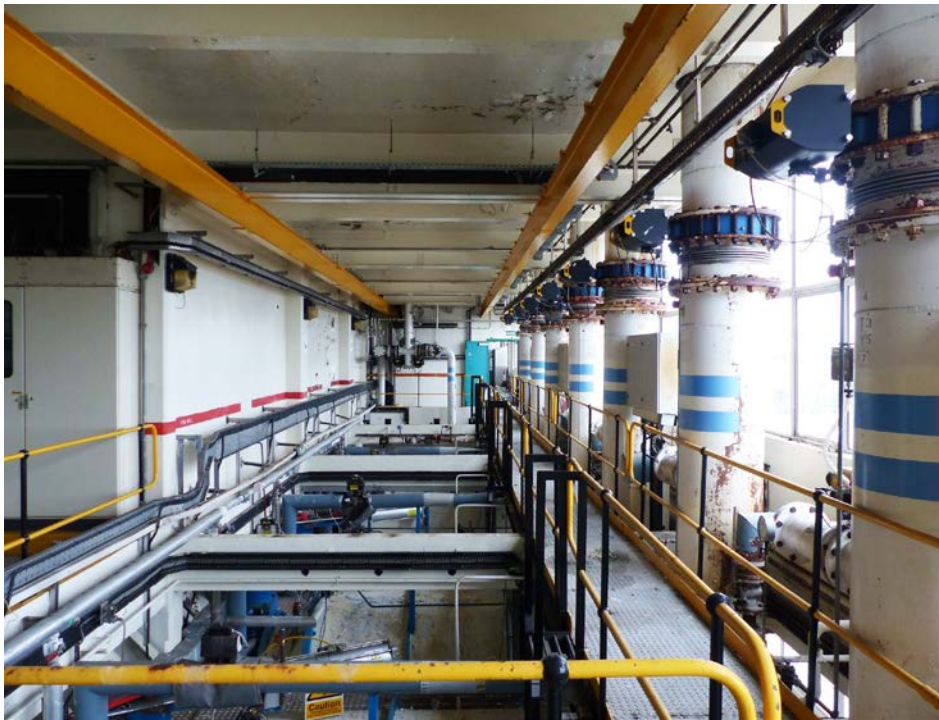
Fig 61 Food production area in the north-east corner of the third floor, looking north
