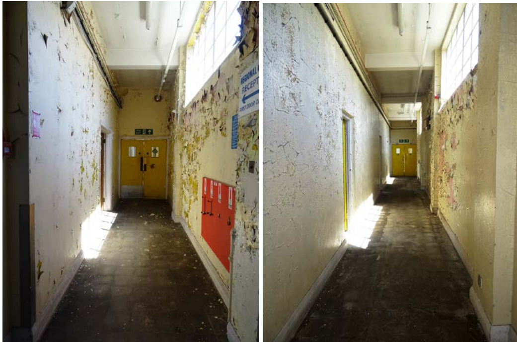
Fig 79 South end (left) and a central portion (right) of the north-south running corridor on the first floor of the west wing.
