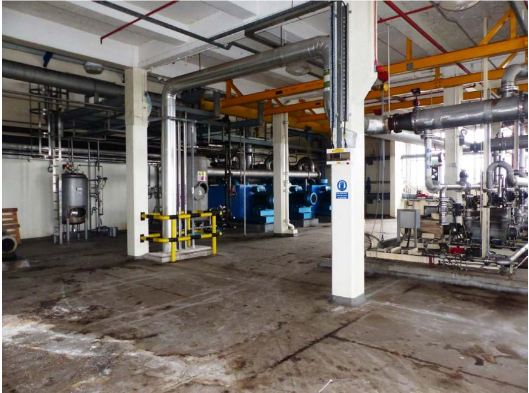
Fig 63 Plant and machinery along the north end of the third floor
