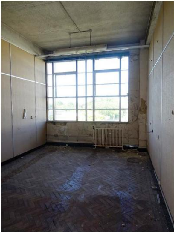
Fig 81 One of the first-floor office rooms in the west wing with herringbone wood parquet flooring
