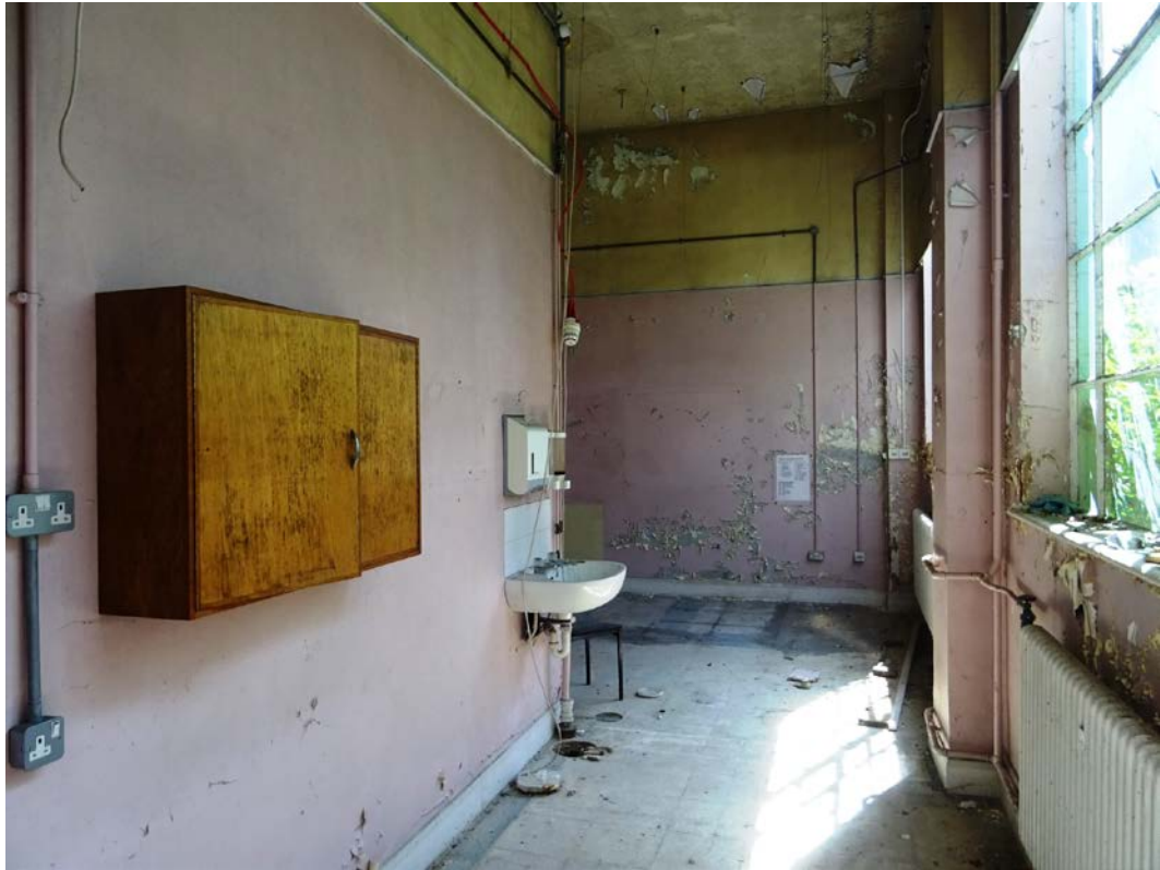
Fig 74 Kitchen area at the east end of the south wing, looking east
