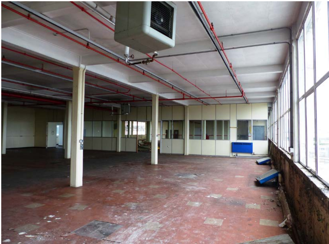
Fig 57 Storage areas in the south-east section of the third floor (3F9), looking north-west
