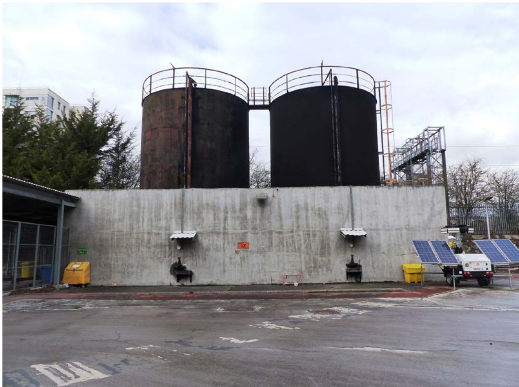
Fig 150 A couple of large tanks along the north-west boundary of the site along the canal, looking north
