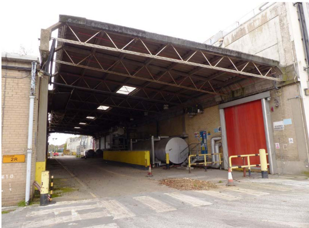
Fig 24 Loading bay covered in a canopy at the northern end of the east elevation
