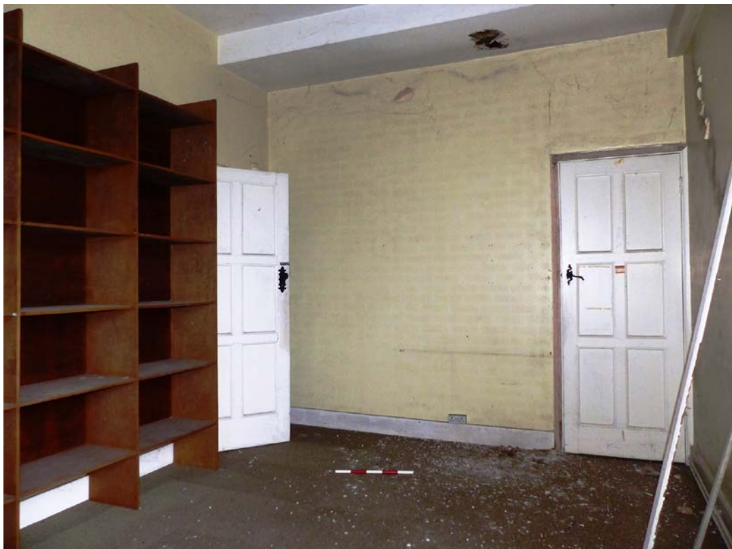
Fig 104 Room G6, looking south-west. Note door to the former pantry on the right
