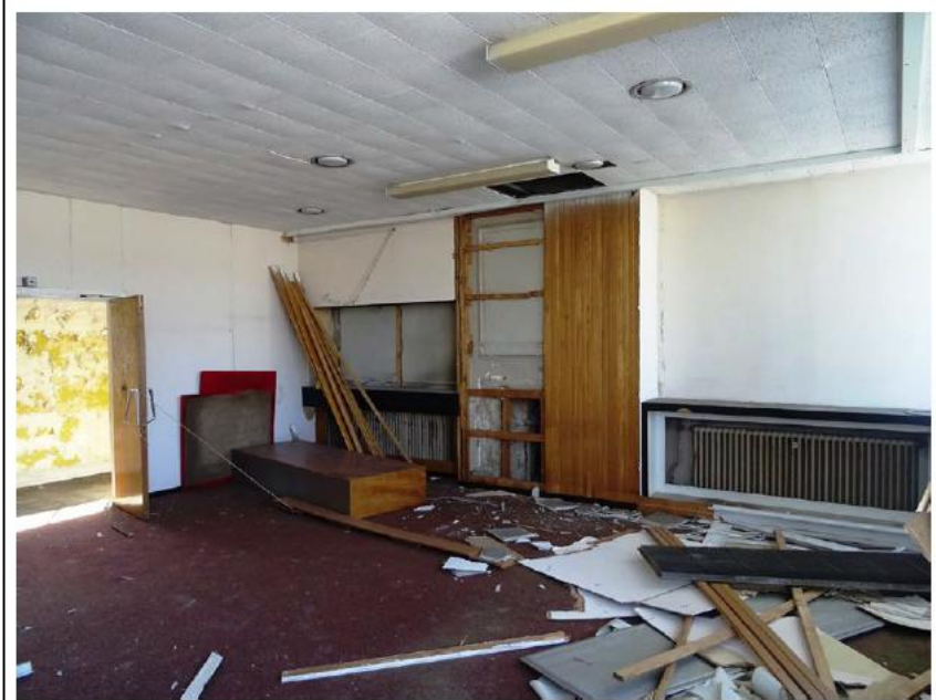
Fig 80 Southern end office room on the first floor of the west wing, looking south-east
