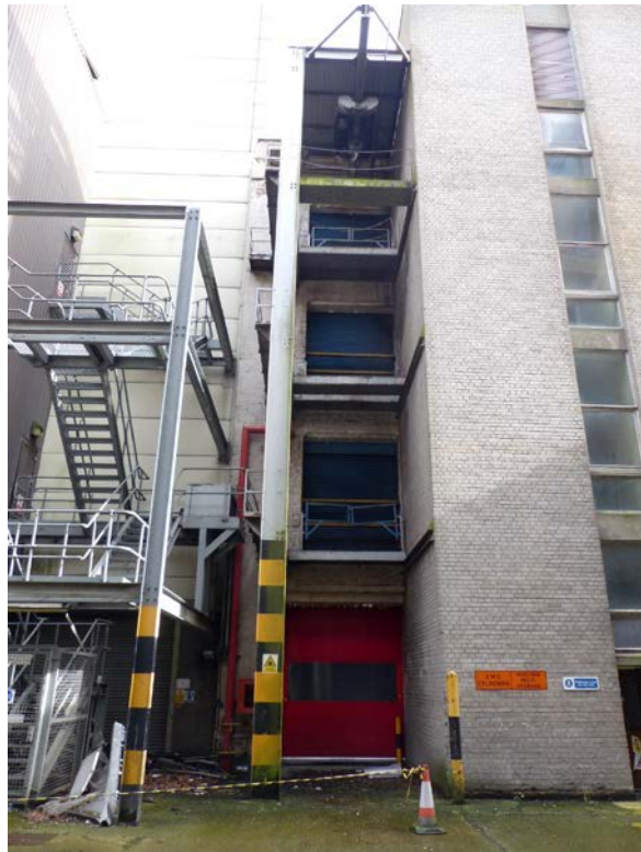
Fig 20 Loading platforms have been added to the north end of the west elevation. Loading bays have been formed by inserting openings in the older part of the factory
