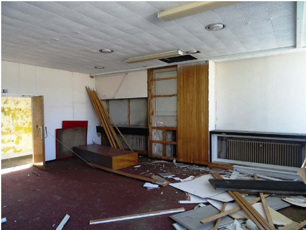
Fig 80 Southern end office room on the first floor of the west wing, looking south-east
