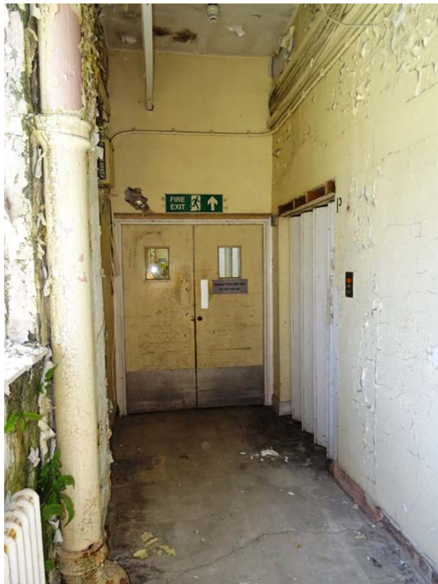
Fig 83 Goods lift accessed from the corridor on the first floor
