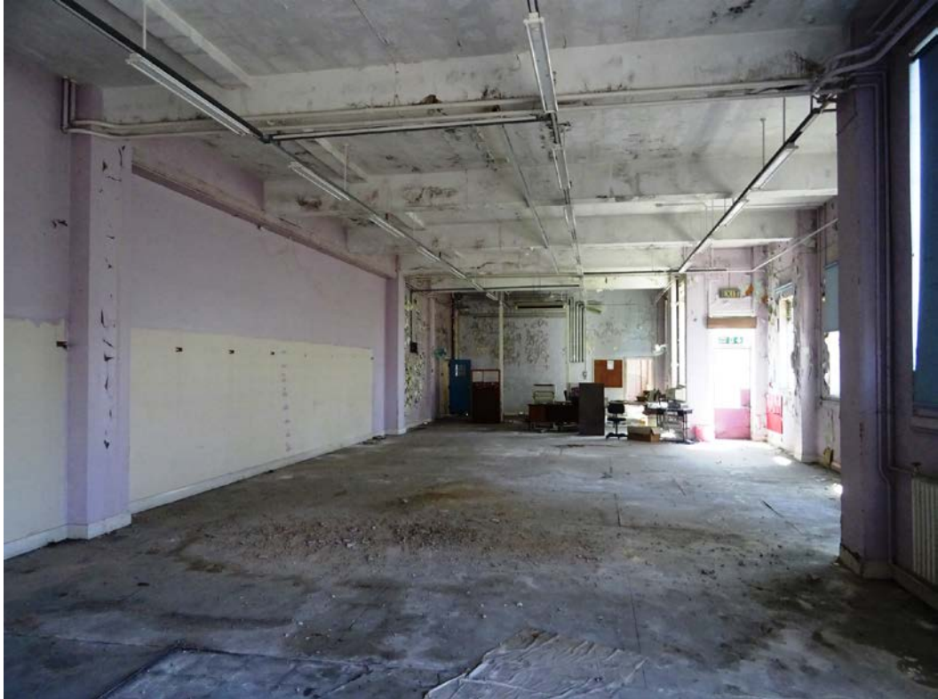
Fig 73 The main office area in the south wing on the ground floor, looking east
