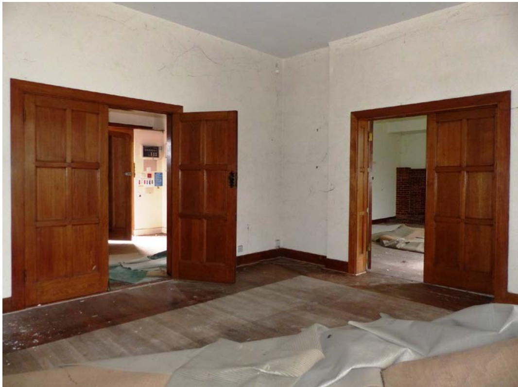
Fig 96 Room G2. Note double timber doors to the stairwell and to room G5, looking north-east
