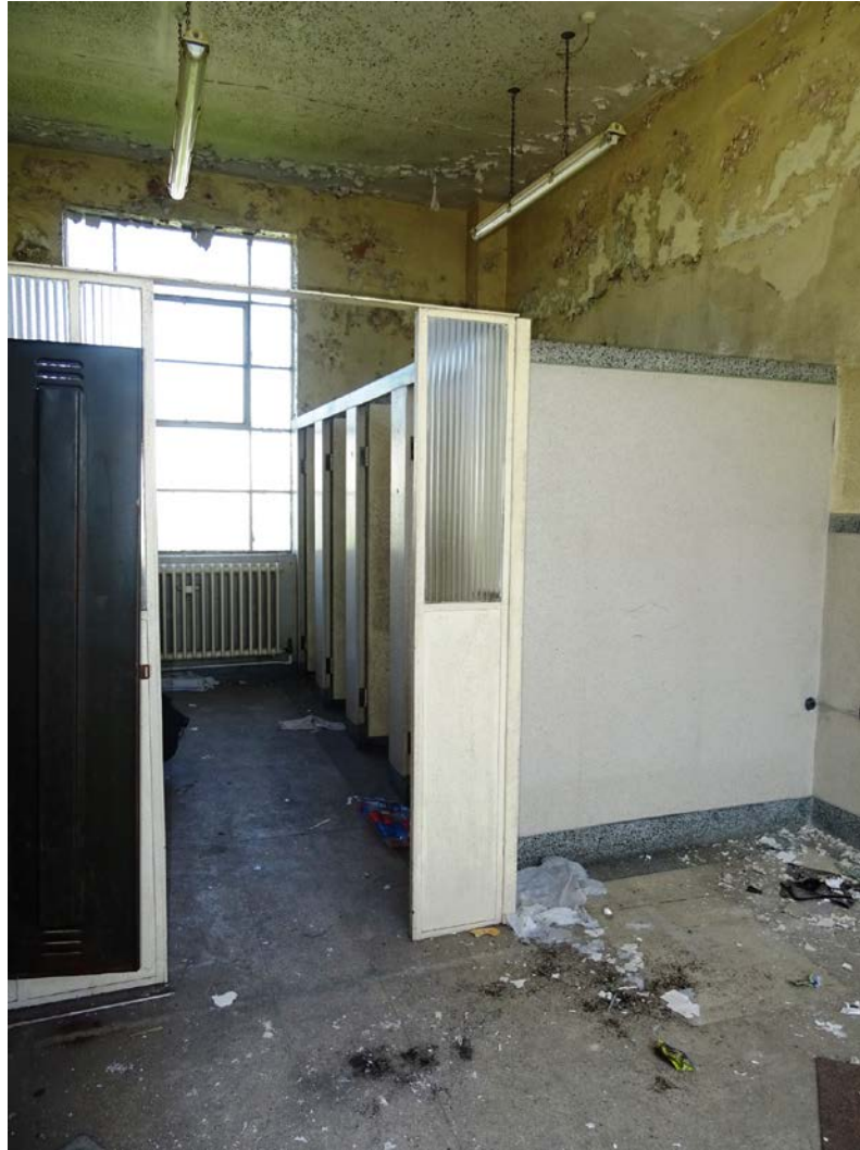
Fig 84 Female WC in the northern end of the west wing on the first floor
