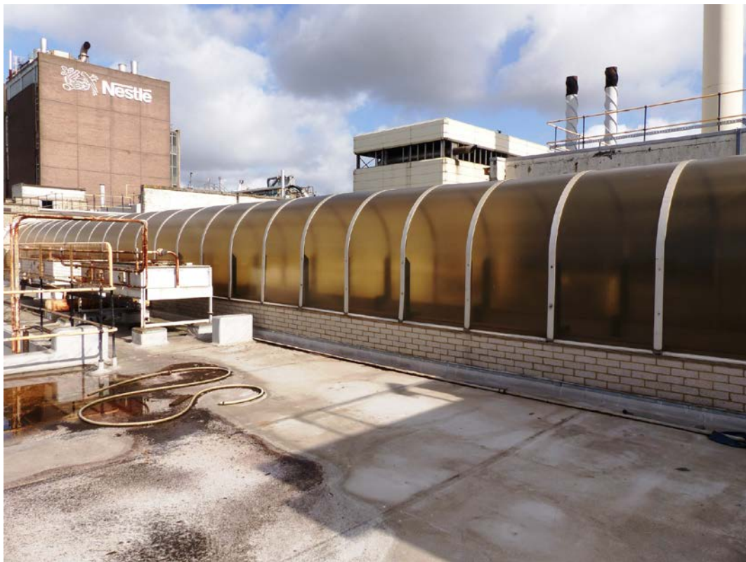
Fig 58 Covered walkway providing access to the older part of the building on the third floor
