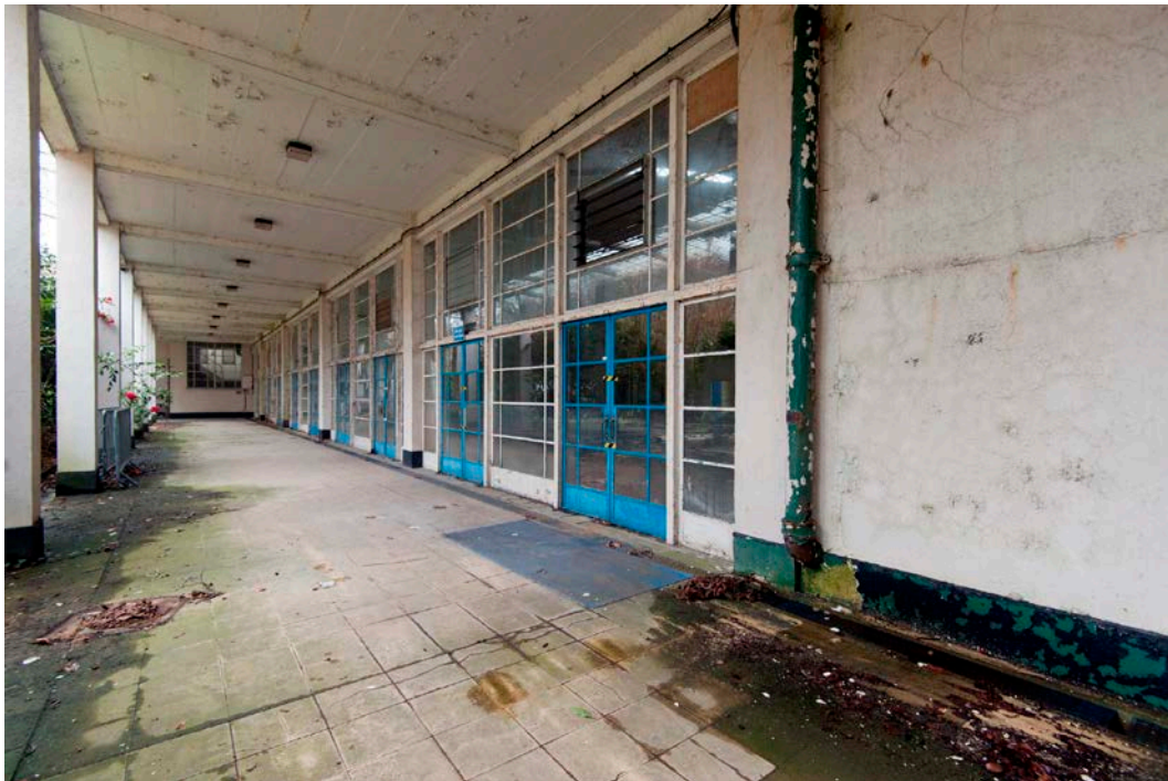
Fig 70 East elevation of the main hall and the interior of the colonnade, looking south-west
