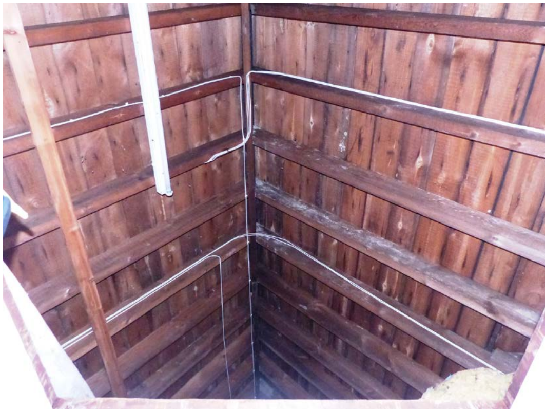
Fig 114 Common rafter timber boarded roof construction was visible through a hatch in the ceiling of room 2F2
