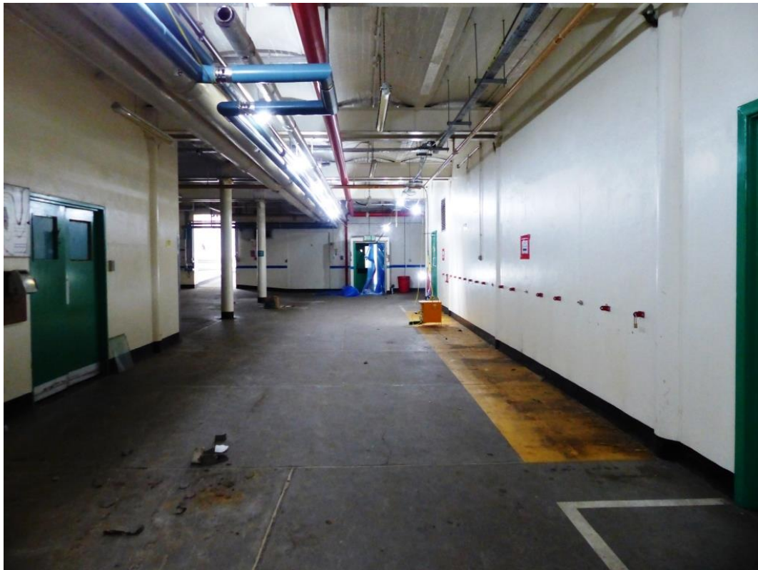
Fig 49 Evidence of the original 1914 Sandow building looking west; the doors to room 1F32 can be seen in the left of the photograph.
