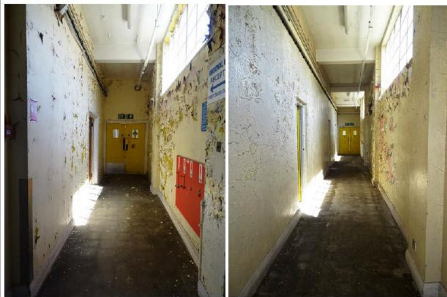
Fig 79 South end (left) and a central portion (right) of the north-south running corridor on the first floor of the west wing.
