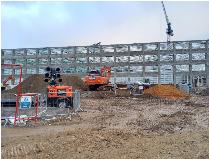
Service yard area to front of Unit 4
