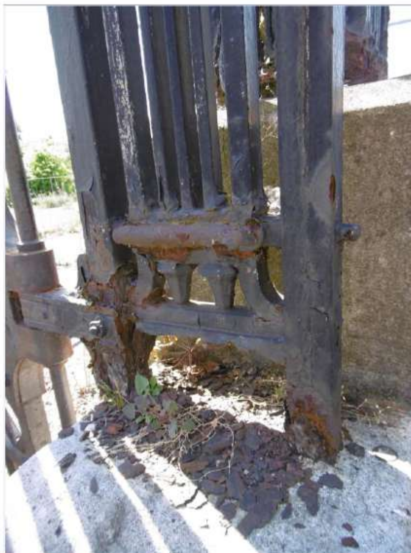
Fig 11: Western gate corner post, corrosion exposed
