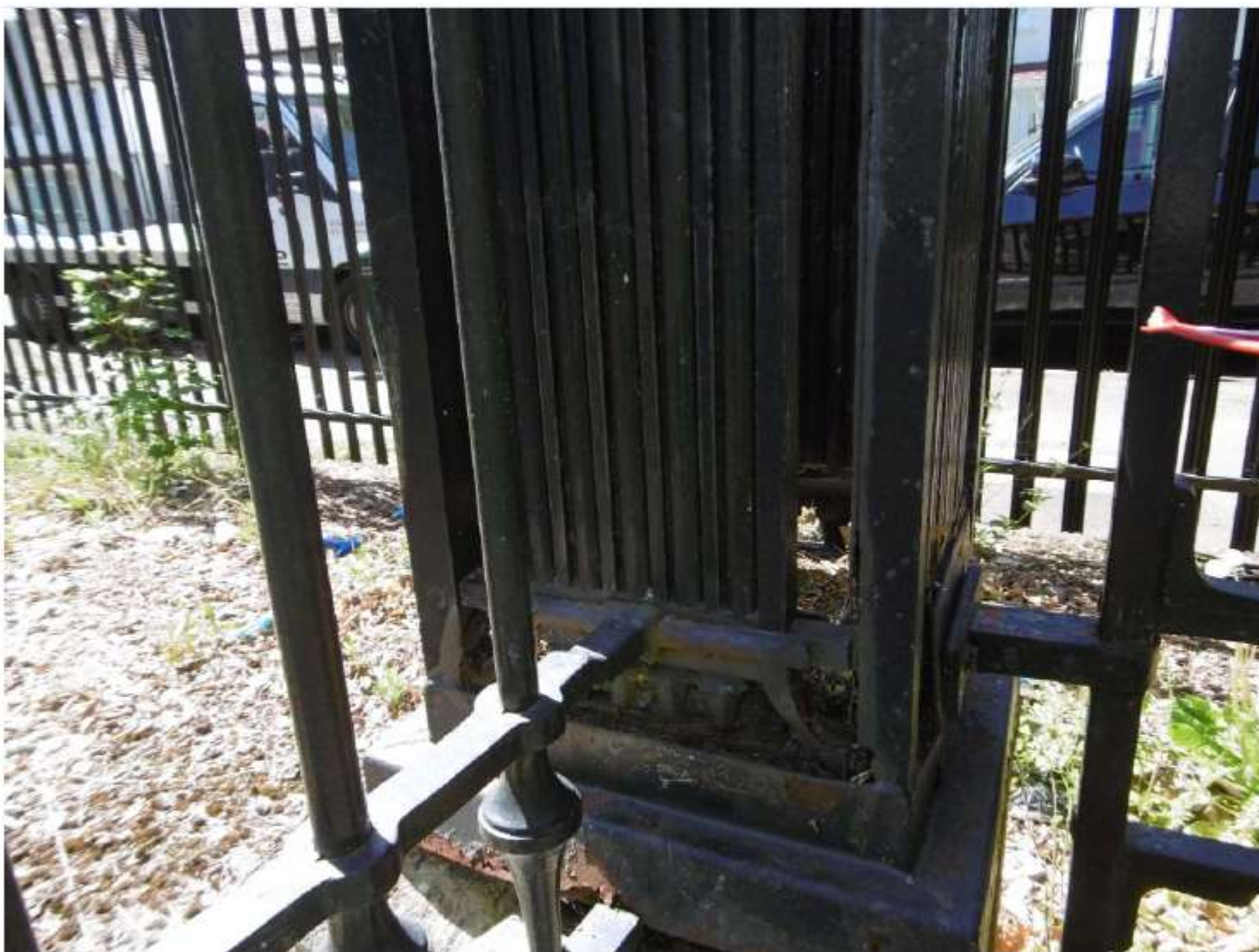
Fig 2: Central gate corner post looking south, base showing exposure and corrosion
