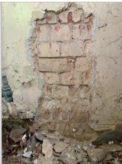
P1e: DPC INVESTIGATION - SURVEY AREA RR13
