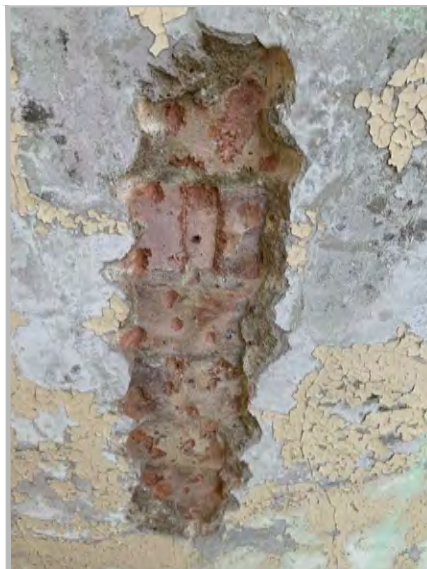
P1f: CRACK INVESTIGATION - SURVEY AREA RR3
