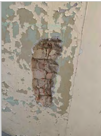
P1g: CRACK INVESTIGATION - SURVEY AREA RR4
