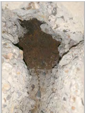
P3b: CLOSE UP VIEW OF PRIMARY BEAM A-C/9
