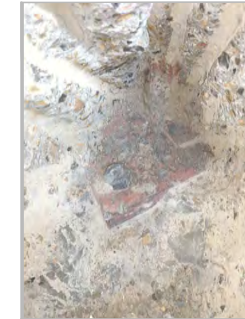
P18b: CLOSE UP VIEW OF EXPOSED BASE PLATE TO COLUMN J3
