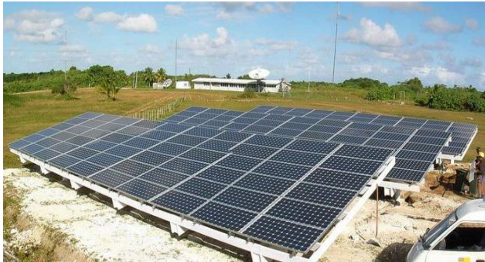
Figure 8.2: Photovoltaics 30kW peak PV Installation
