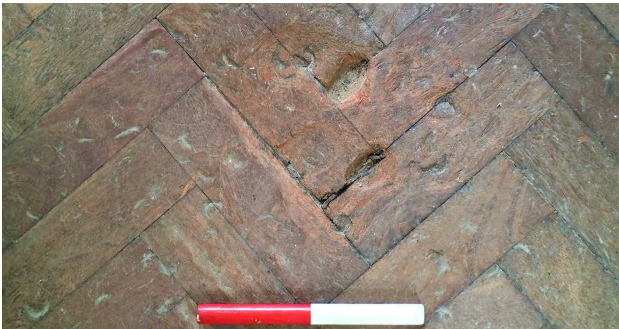
Fig 63 Gouges in the parquet flooring caused by the stools
