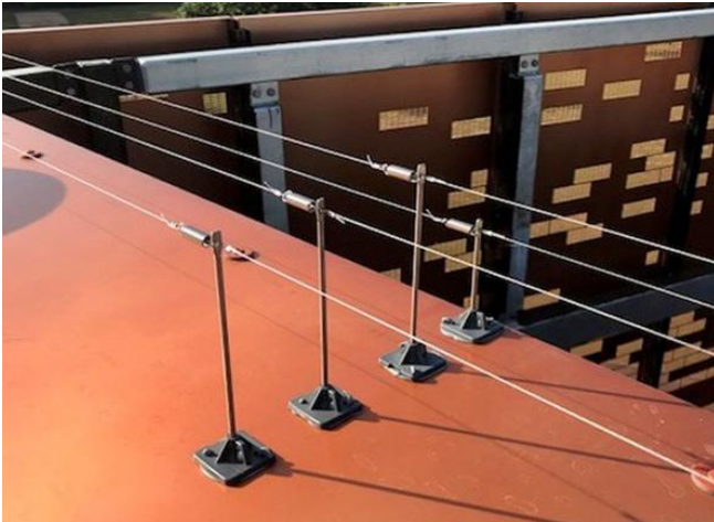
Plate 3.2 Bird Spike Control : bird trip wire
