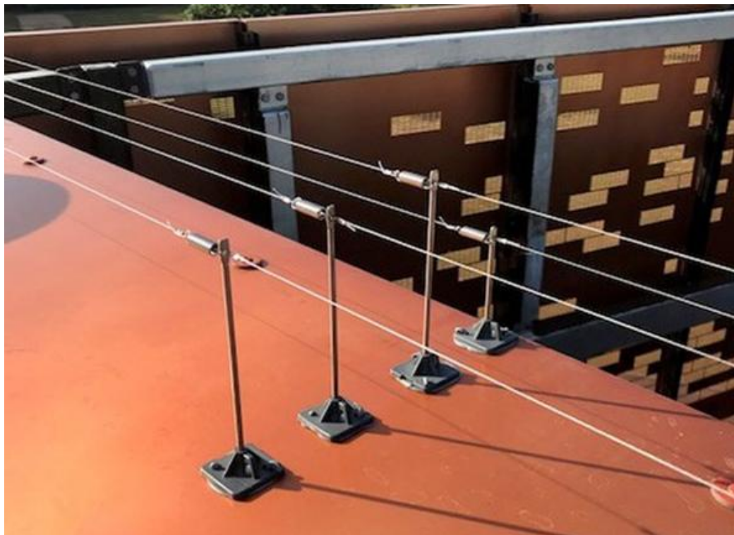
Plate 3.1 Bird Spike Control: bird trip wire
