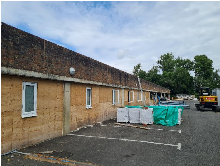
Plate C.4 Newly created rooms within the lower car park level, functioning as contractor office space and welfare facilities.
