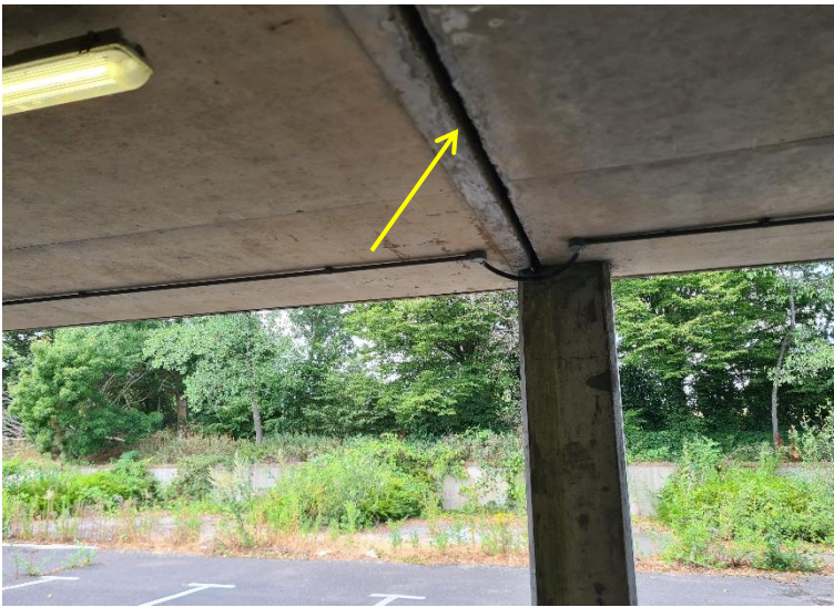
Plate C.11 Linear ceiling gap viewed from the lower car park level.
