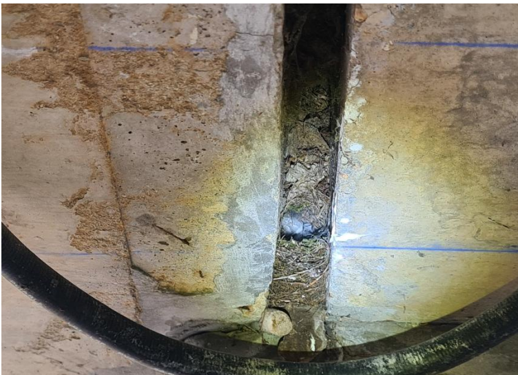
Plate C.12 Bird nest locating between adjoining roof sections of the car park.
