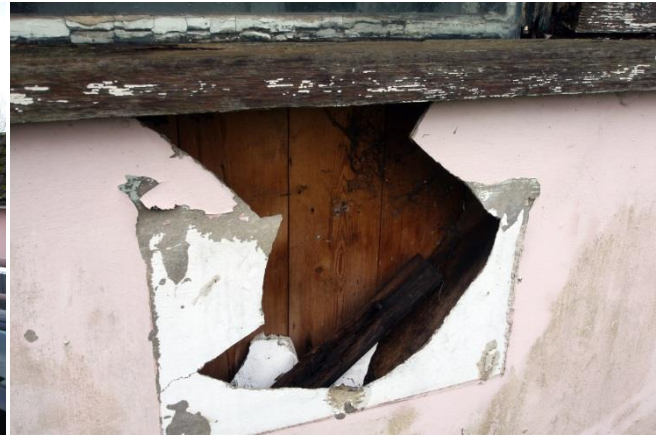
Damaged asbestos cement cladding with no insulation
