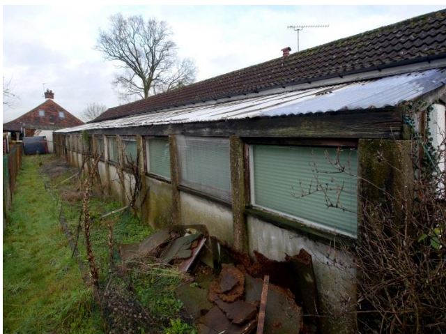
Side view of lean-to shows poor construction and very poor condition with non-fire rated corrugated plastic roof. This is a part of the house footprint and referred to as a conservatory.
