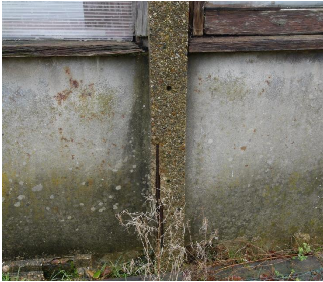
Lean-to. Structural Concrete post with exposed reinforcement.
