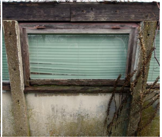
Rotting timber windows. Posts are not vertical and are unrestrained at the head
