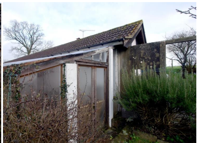
End panel infill in timber supports the collapsing structure
