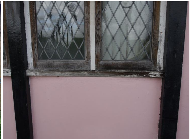
Rotting timber framed windows set between the concrete posts and over concrete panel. Render is loose and bulging.
