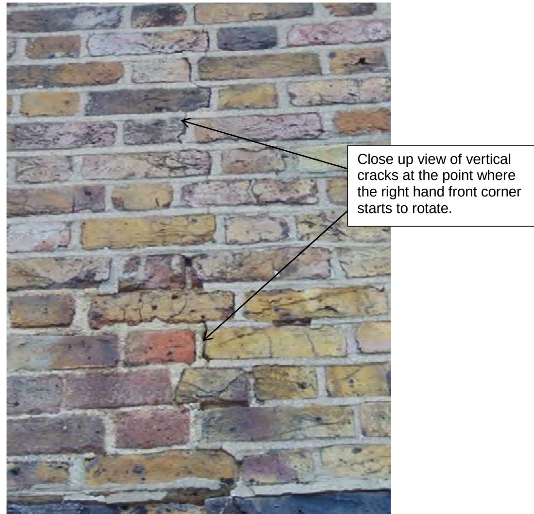
Figure 19 showing vertical cracks that appear in several places along the West elevation masonry
