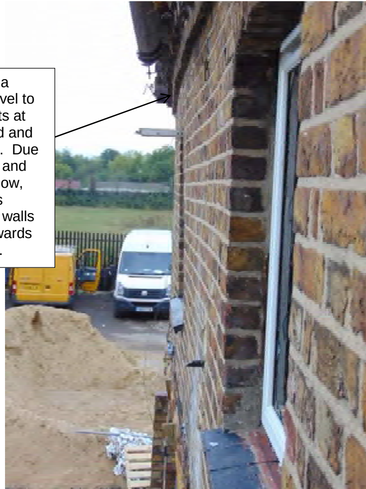
Figure 28 showing the degree of bulge in the rear masonry wall
