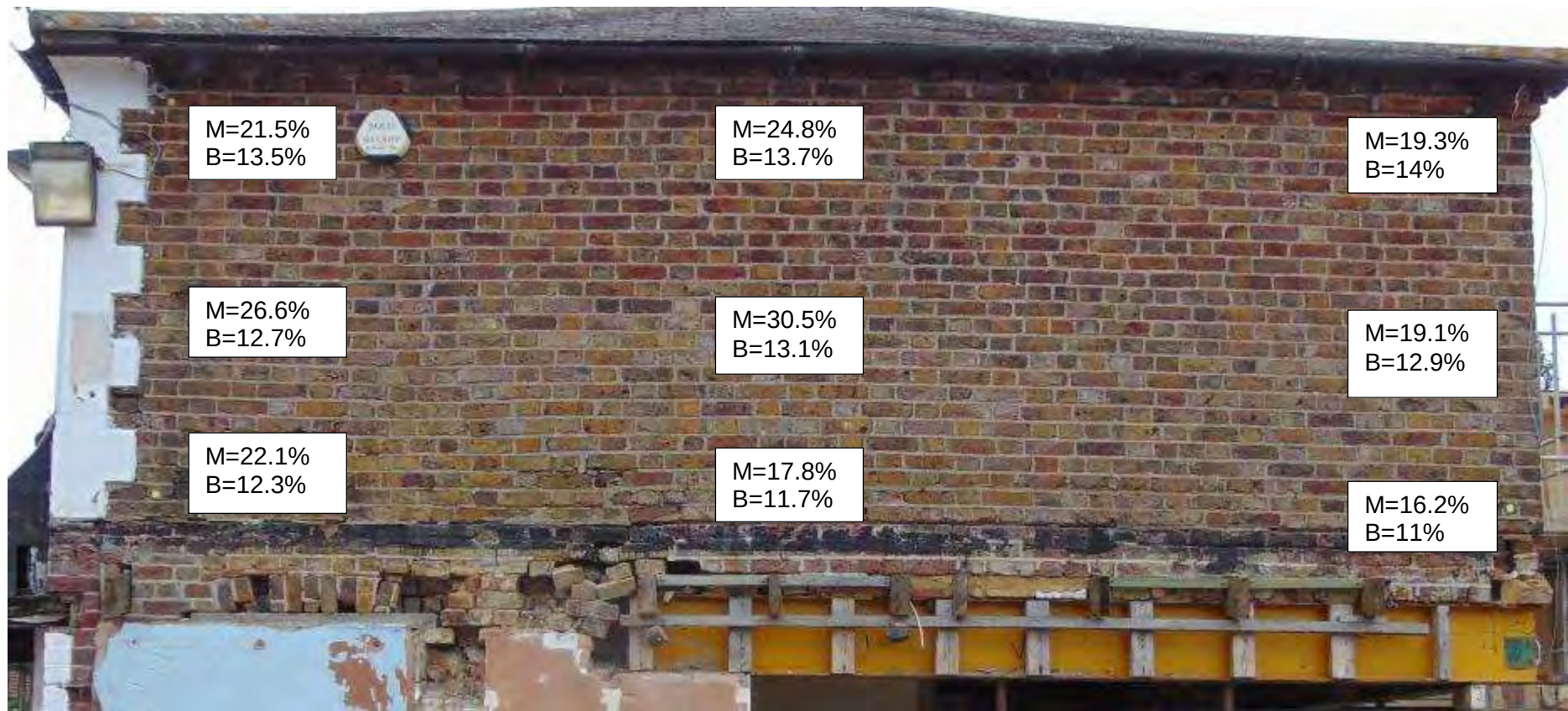
Figure 13 showing moisture content in the mortar (M) and the bricks (B) at set points across the elevation
