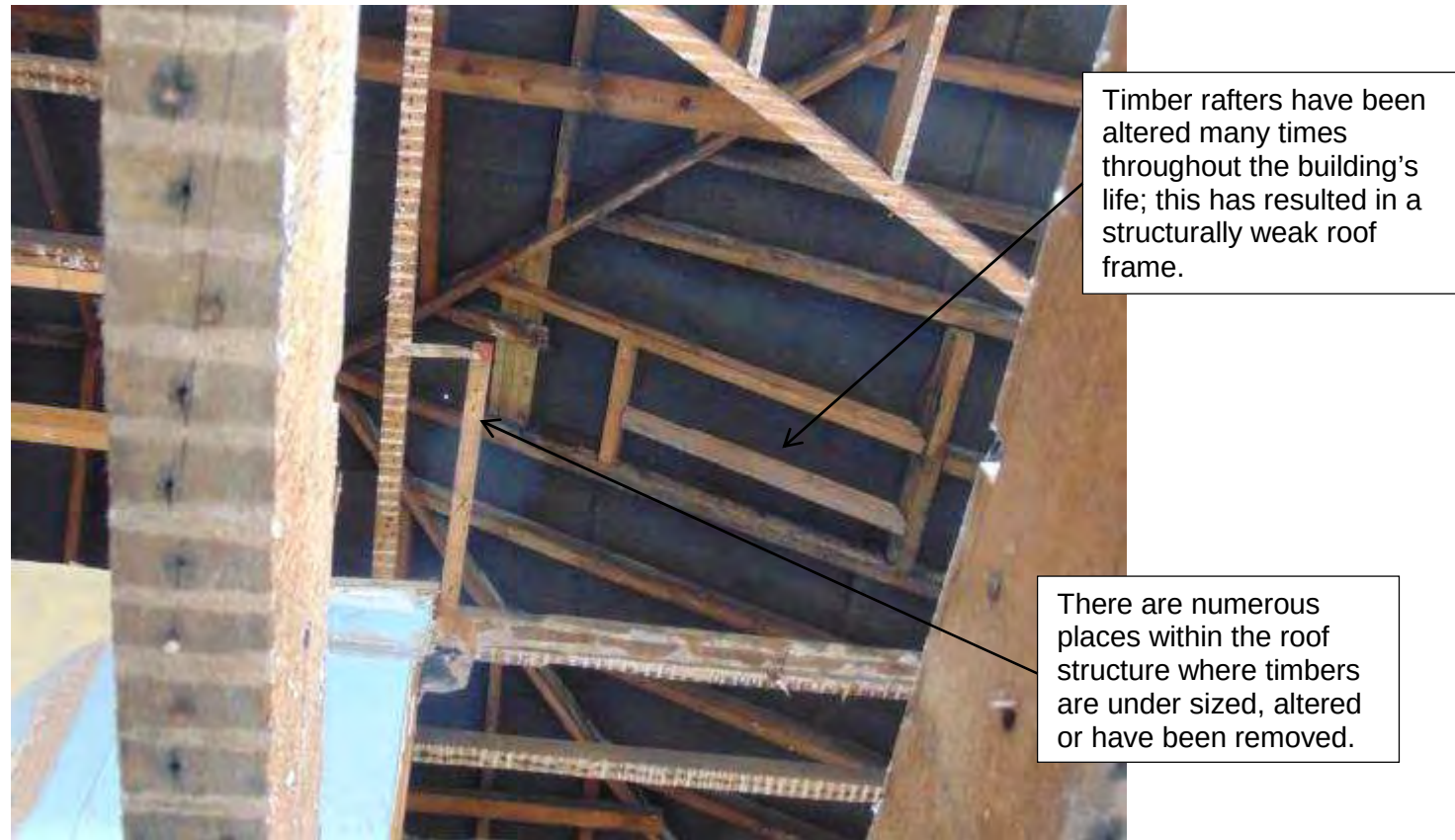
Figure 31 Close up of under sized and altered/missing joists and rafters
