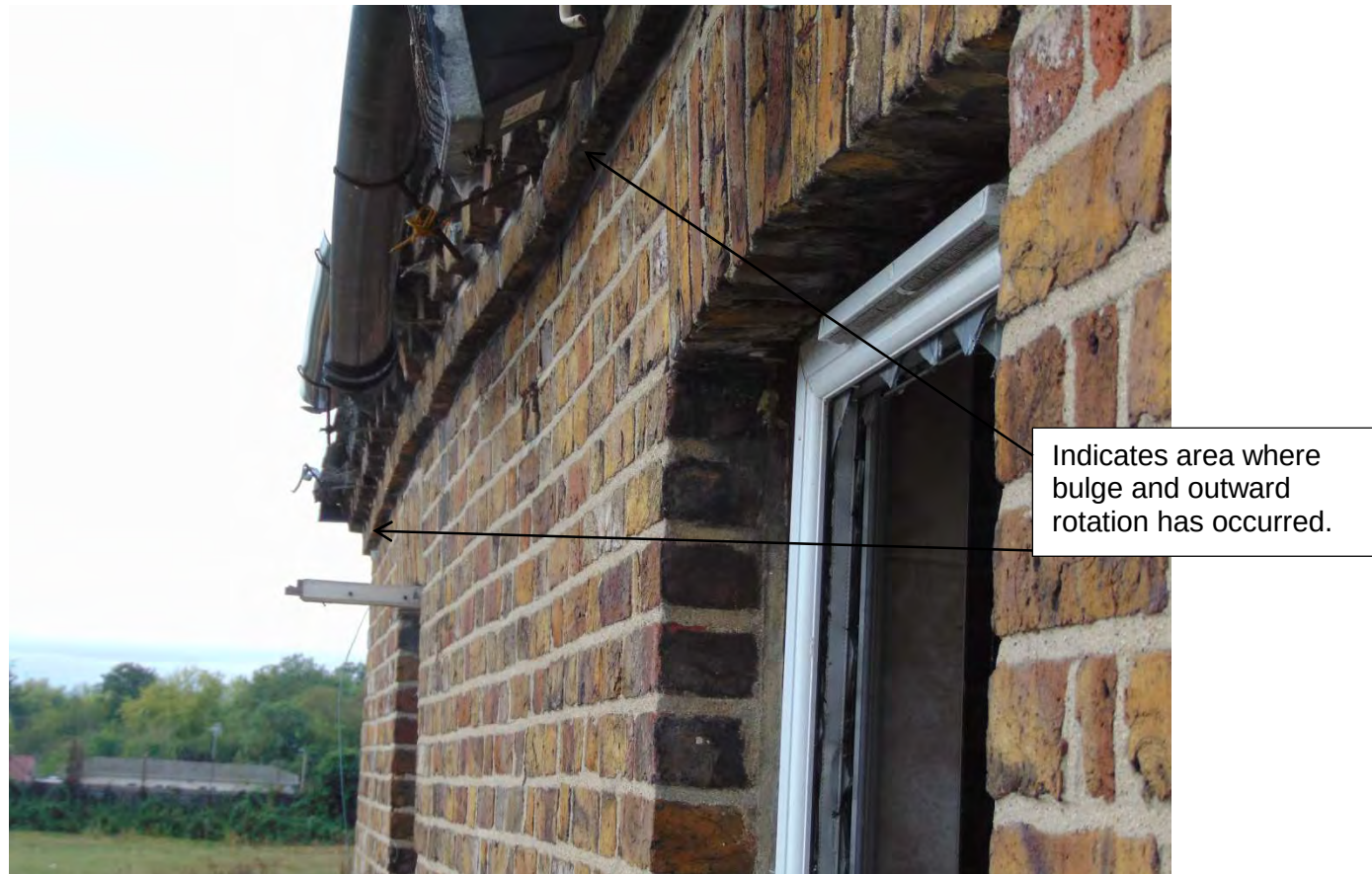
Figure 29 showing the distance that the masonry wall to the rear bulges outwards
