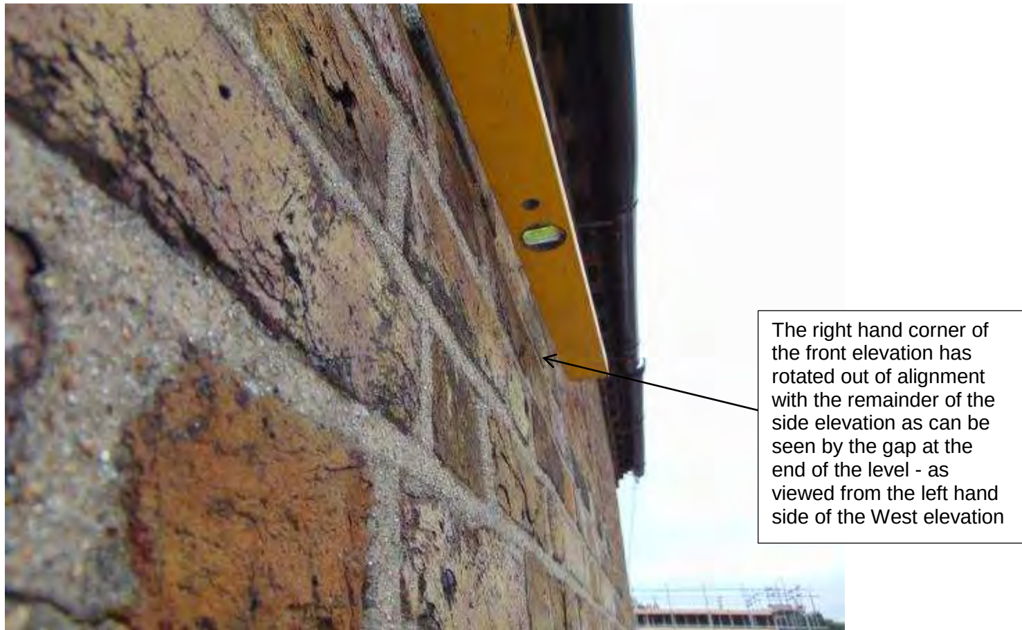
Figure 17 showing how the left hand corner of the West elevation wall has rotated out of alignment with the remaining wall
