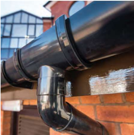
MARLEY UPVC DEEPFLOW RAINWATER GUTTER AND RAINWATER DOWN PIPE FIXED TO WOODGRAIN UPVC FASCIA COLOUR : BLACK
