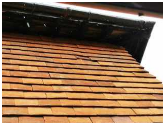
Photo 2. Gaps beneath hanging tiles on Building 1.
