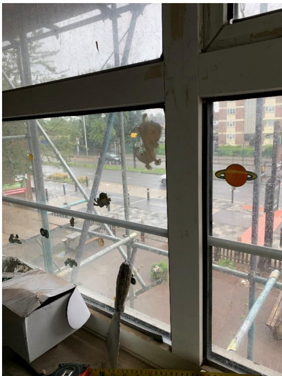
Image 2 Existing PVCu Windows
