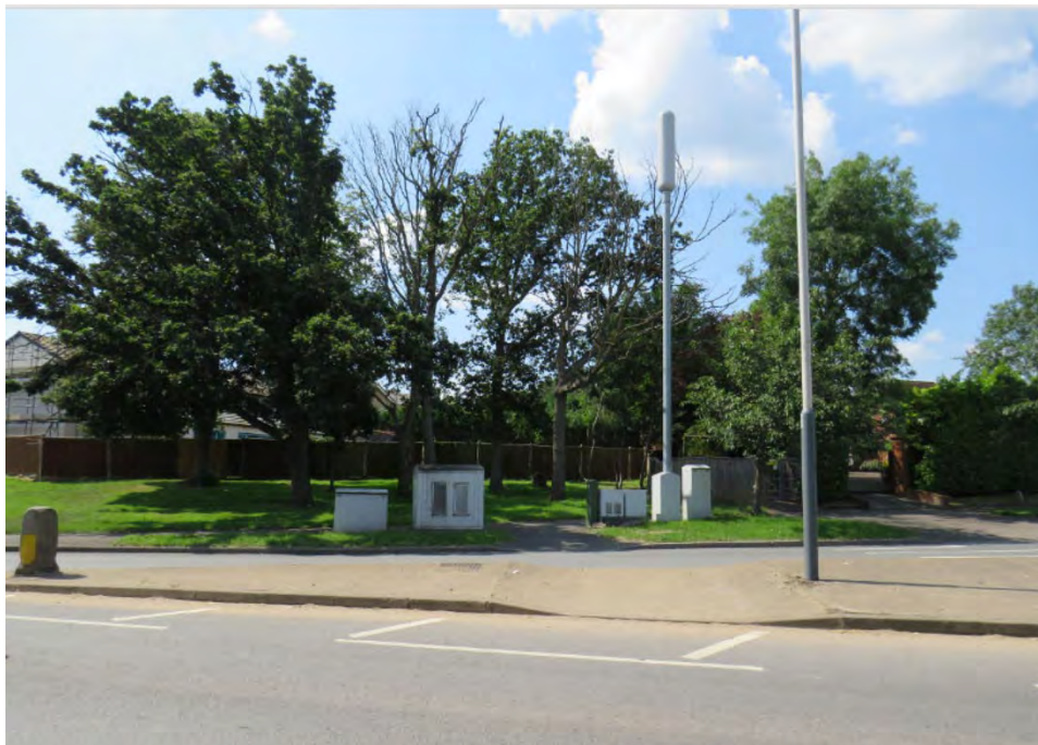
Photograph No. 2 – Existing telecommunications site on Swakeleys Road / Havril Road roundabout
