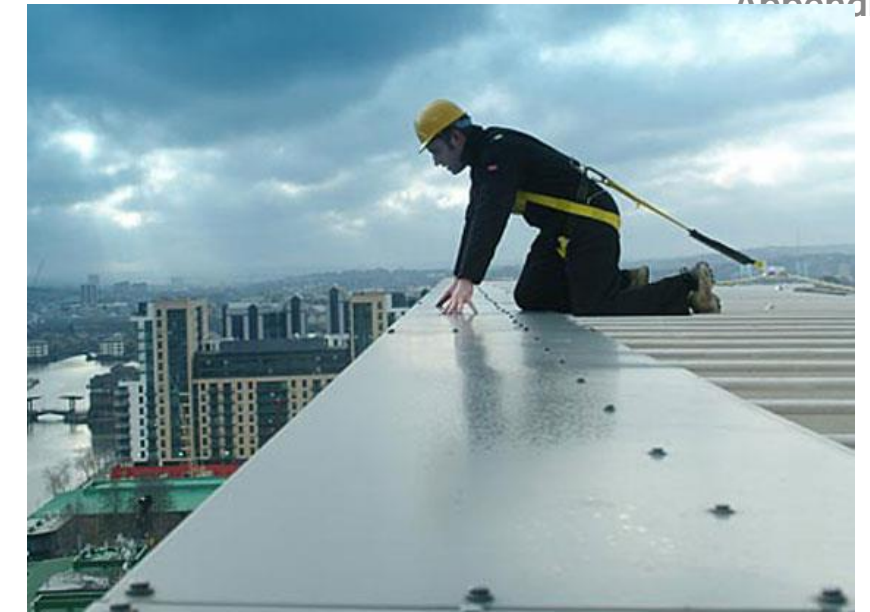
Figure 25 – Typical Safety Line system
