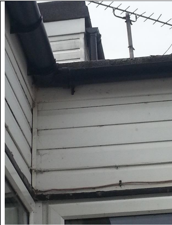
Photograph 13. TN3- gaps beneath bitumen felt on roof.
