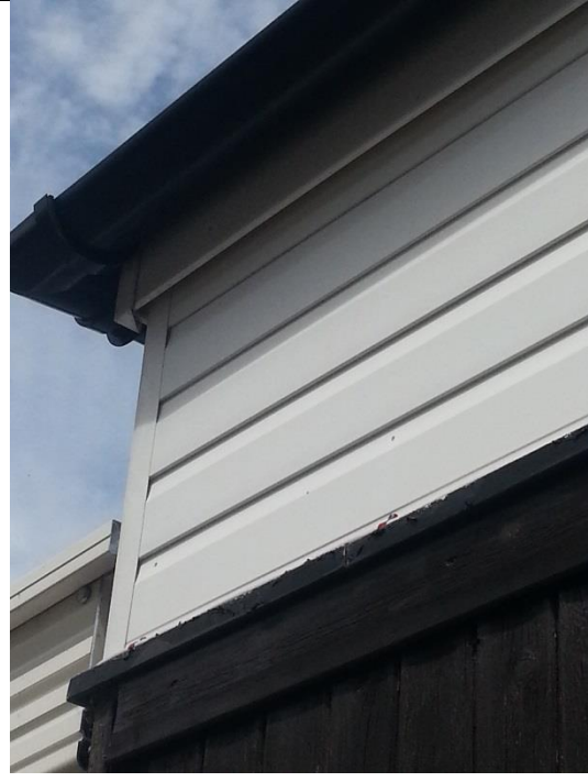
Photograph 12. TN2- Example of gaps underneath soffits.
