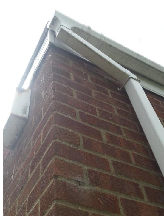
Photograph 14. TN4- slight gapping between soffit box and wall.
