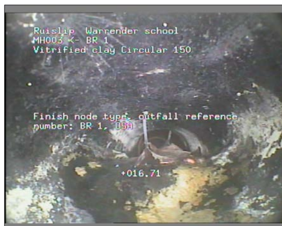
Photo: 7_7_28_A.JPG 16.68m, Deformed sewer/drain, 60%
