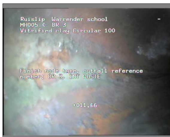
Photo: 16_16_65_A.JPG 11.66m, Finish node type, outfall reference number: BR 3
