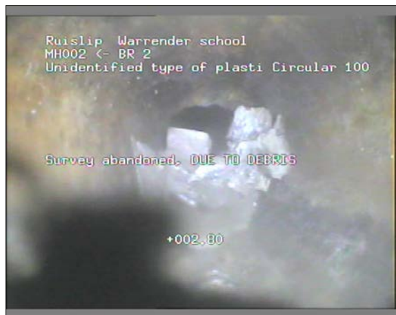
Photo: 4_4_14_A.JPG 2.8m, Settled deposits, hard or compacted, 70% cross-sectional area loss
