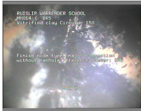
Photo: 52_52_201_A.jpg 2.34m, Finish node type, major connection without manhole reference number: BR5
