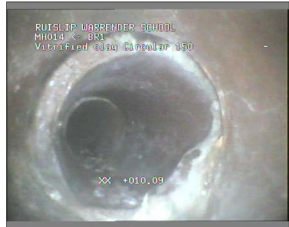
Photo: 48_48_183_A.jpg 10.09m, Joint displaced, medium
