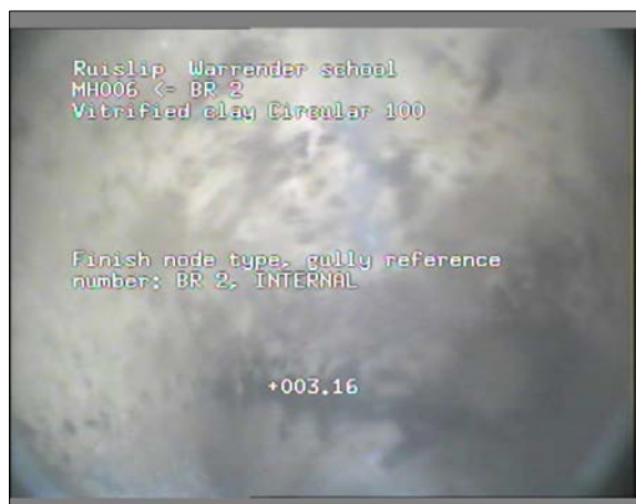
Photo: 24_24_99_A.JPG 3.16m, Finish node type, gully reference number: BR 2
