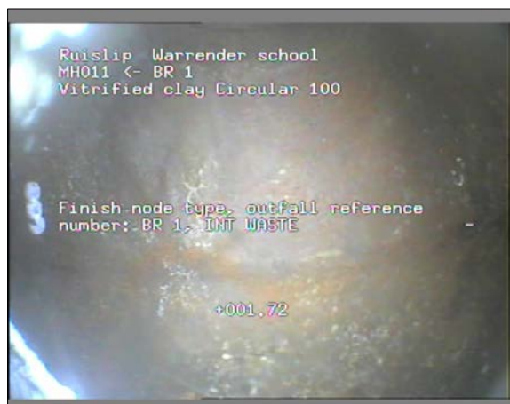
Photo: 27_27_110_A.JPG 1.72m, Line deviates up
