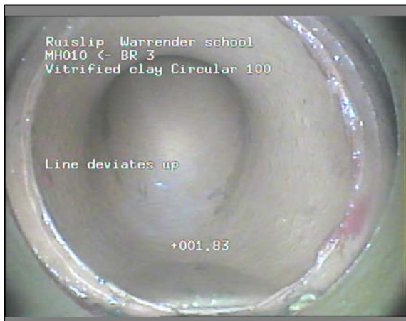
Photo: 31_31_123_A.JPG 1.83m, Line deviates up
