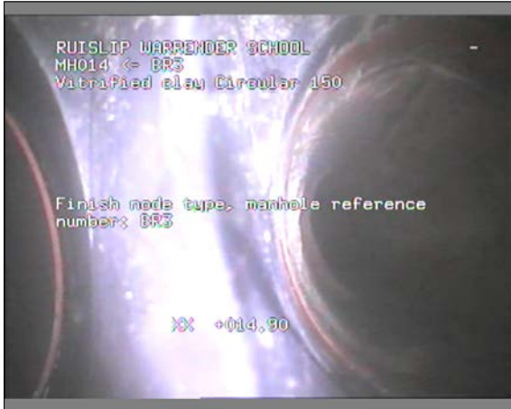
Photo: 50_50_194_A.jpg 14.9m, Finish node type, manhole reference number: BR3
