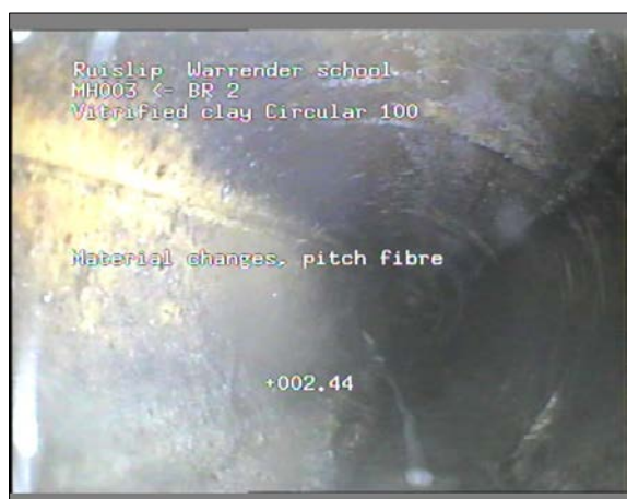
Photo: 8_8_32_A.JPG 2.44m, Material changes, pitch fibre
