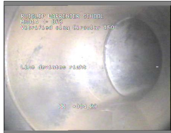
Photo: 50_50_191_A.jpg 4.29m, Line deviates right
