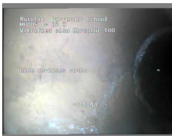
Photo: 16_16_64_A.JPG 11.43m, Line deviates right
