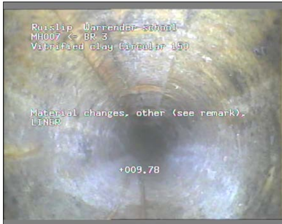
Photo: 20_20_81_A.JPG 9.78m, Material changes, other (see remark)
