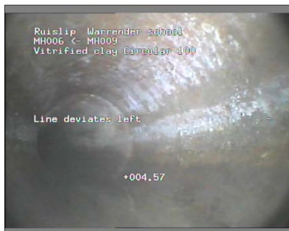
Photo: 22_22_92_A.JPG 4.57m, Line deviates left
