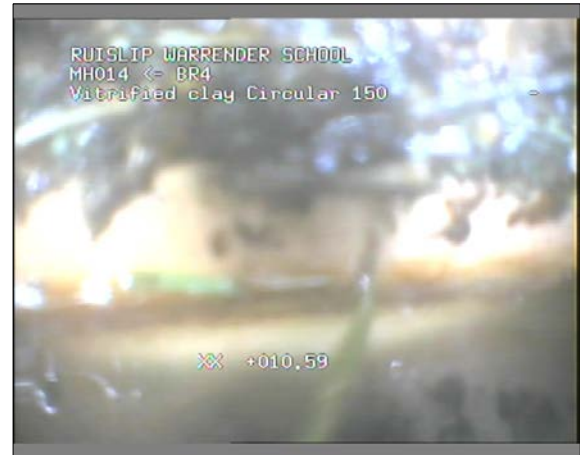
Photo: 51_51_198_A.jpg 10.59m, Finish node type, major connection without manhole reference number: BR4
