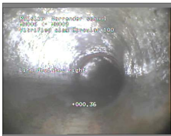
Photo: 22_22_91_A.JPG 0.36m, Line deviates right
