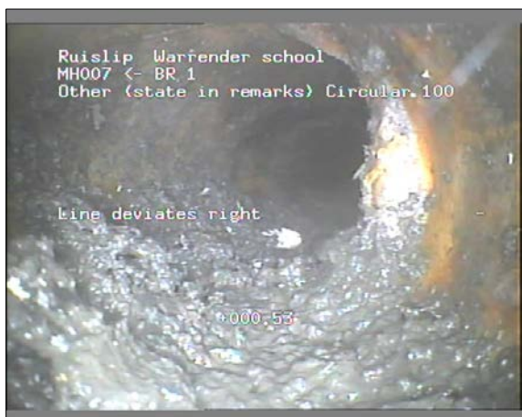
Photo: 18_18_71_A.JPG 0.53m, Line deviates right
