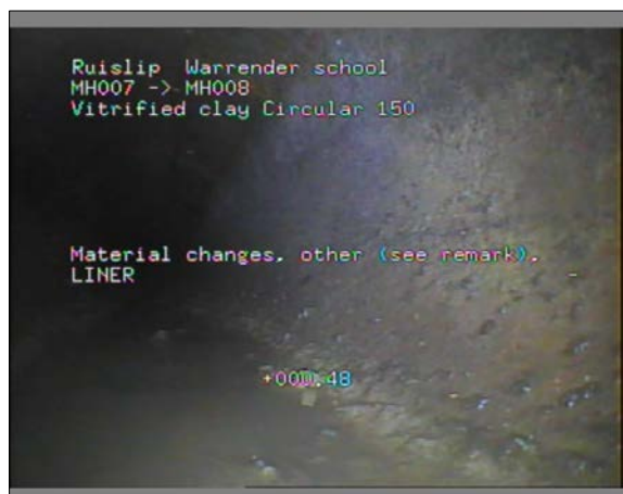
Photo: 21_21_86_A.JPG 0.48m, Material changes, other (see remark)
