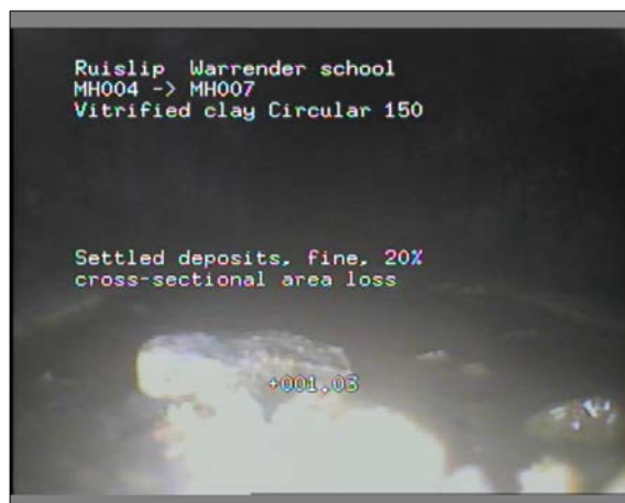
Photo: 13_13_51_A.JPG 1.03m, Settled deposits, fine, 20% cross-sectional area loss
