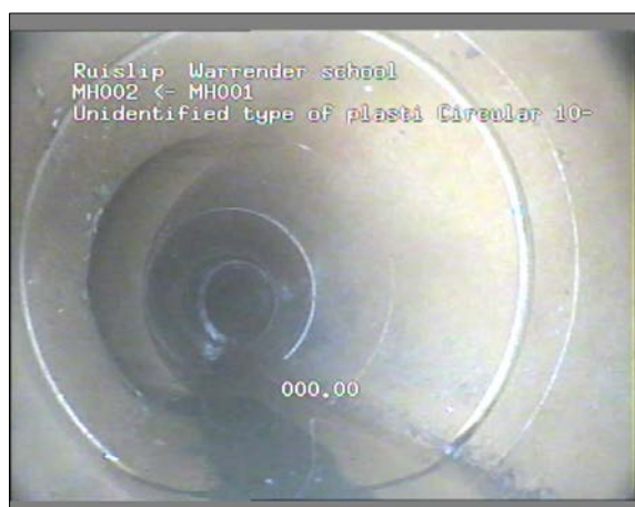
Photo: 1_1_4_A.JPG 0m, Junction, at 9 o'clock, diameter 100mm
