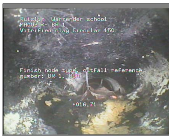
Photo: 7_7_28_A.JPG 16.68m, Deformed sewer/drain, 60%
