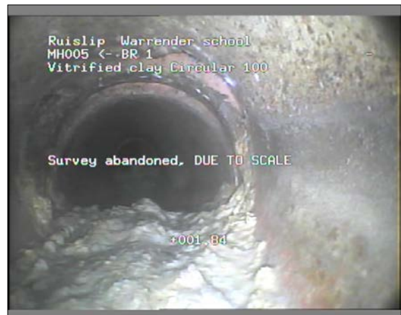
Photo: 14_14_56_A.JPG 1.84m, Settled deposits, hard or compacted, 25% cross-sectional area loss
