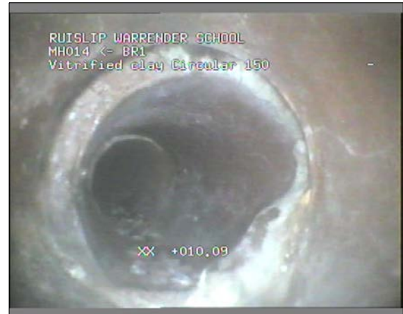
Photo: 48_48_183_A.jpg 10.09m, Joint displaced, medium
