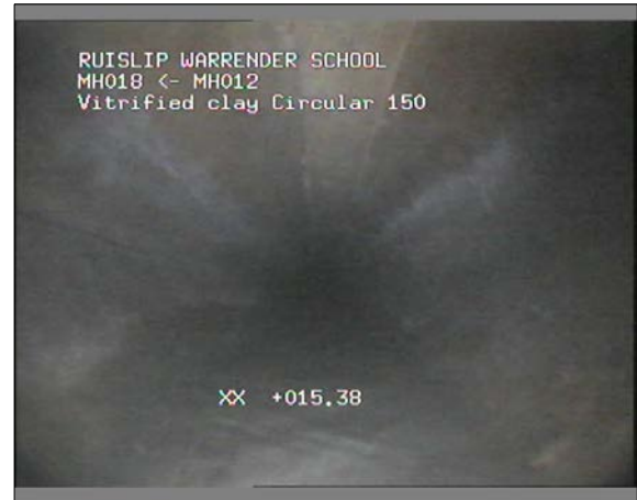
Photo: 53_53_204_A.jpg 15.38m, Finish node type, major connection without manhole reference number: MH012
