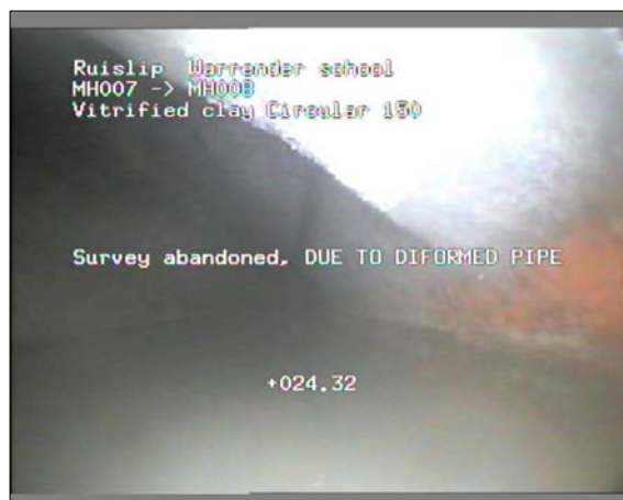
Photo: 21_21_87_A.JPG 24.32m, Deformed sewer/drain, 60%
