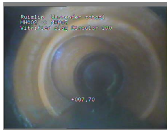
Photo: 5_5_19_A.JPG 7.7m, Junction, at 9 o'clock, diameter 100mm
