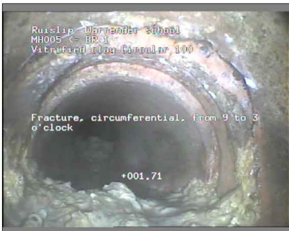
Photo: 14_14_55_A.JPG 1.71m, Fracture, circumferential, from 9 to 3 o'clock
