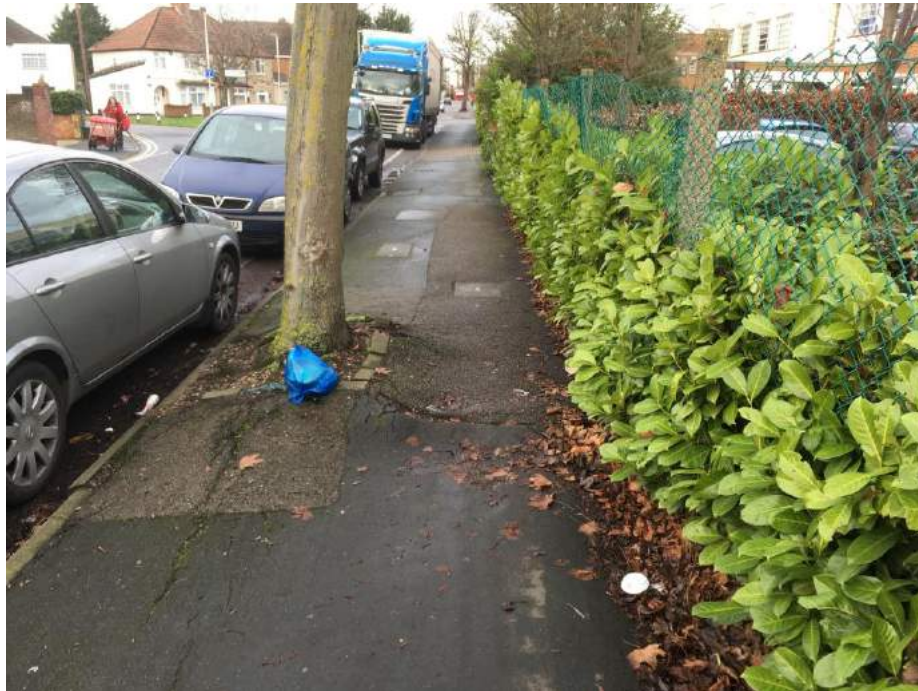
Photo 2 – Trip hazard North Western side of Footway, Nestle Avenue
