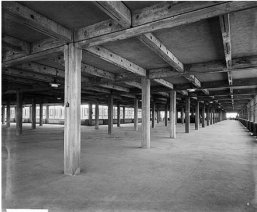
Figure 3.4: Image from 1921 showing the construction of the extension at Hayes Cocoa Factory with exposed concrete beams and posts (Historic England Archives)
