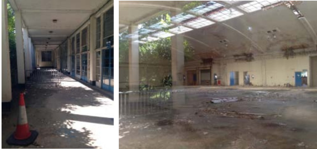
Figure 3.27: (Left) concrete loggia to the east and (right) the vaulted interior of the canteen
