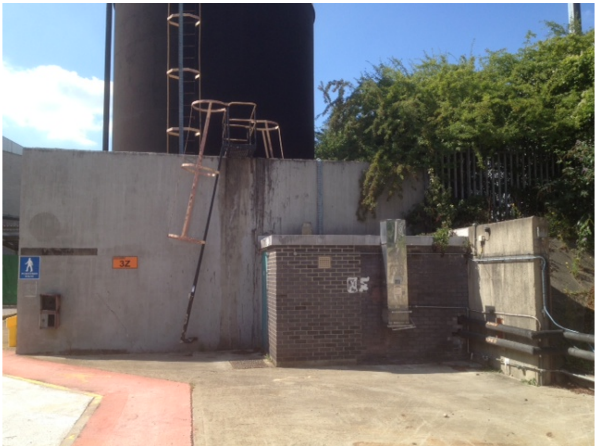
Photograph B2 Diesel AST Bund (from NE)
