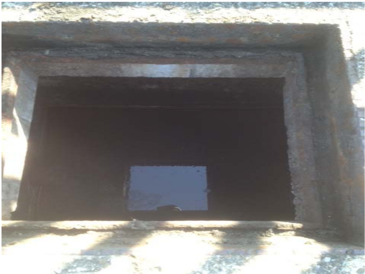
Photograph B6 Water Within One of the Oil-Water Interceptor Chambers
