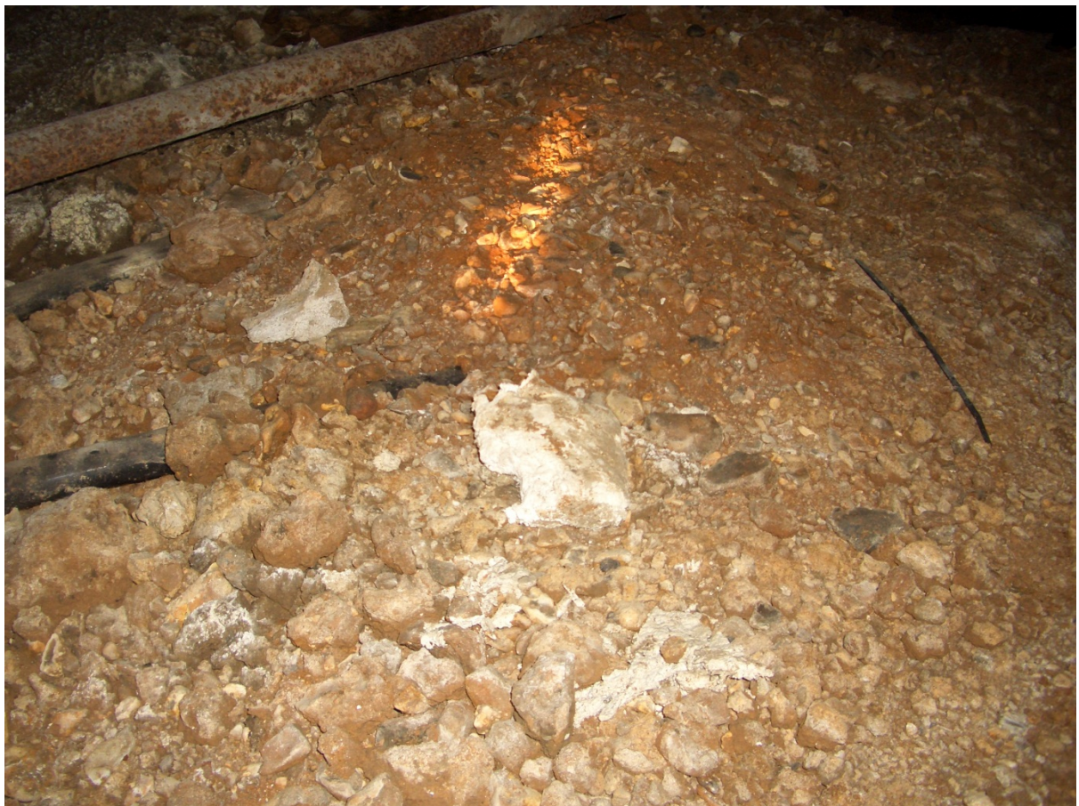
Photograph C8 Undercroft Apparent ACM on Ground
