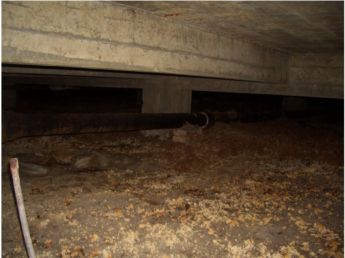
Photograph C7 Undercroft Apparent ACM Lagging on Ground Surface
