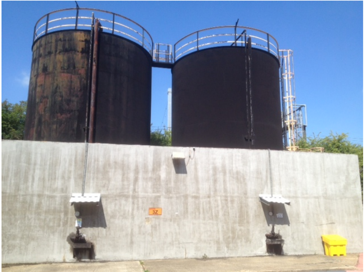
Photograph B1 Diesel AST Bund (from SE)
