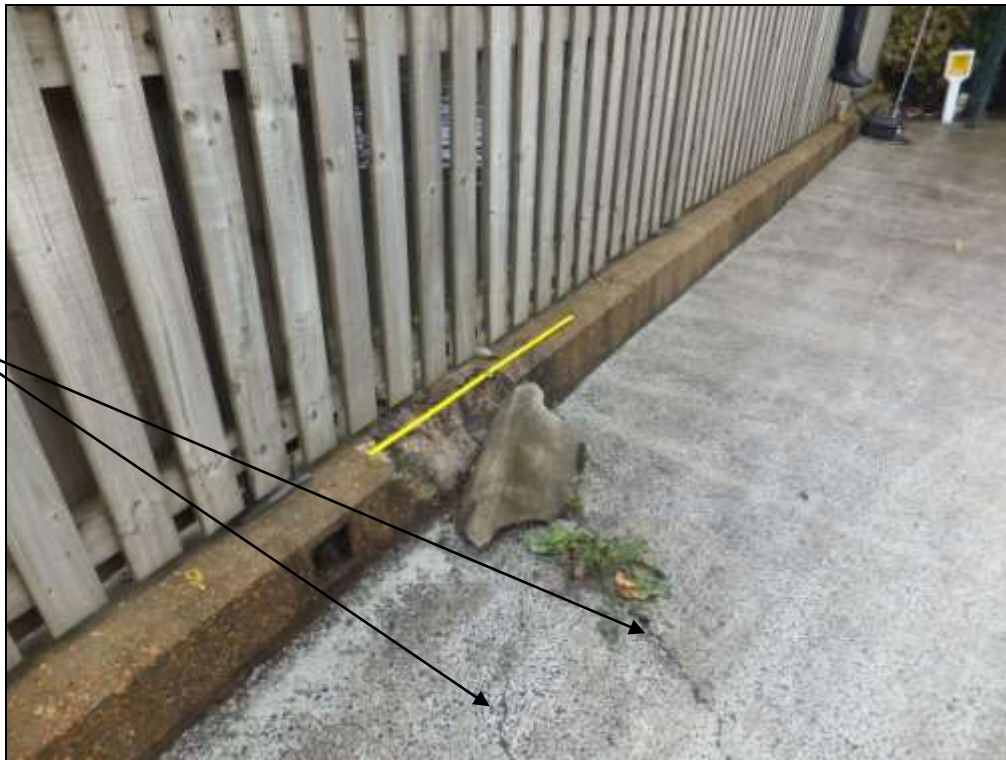
Photograph 7: Ch 40m – Vertical crack running full height of wall.
