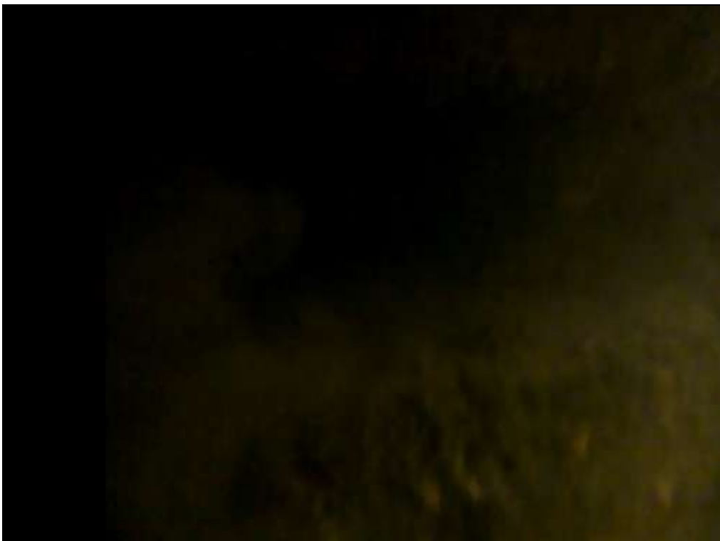
Photograph 40: Ch 280m – Missing brickwork below the waterline.
