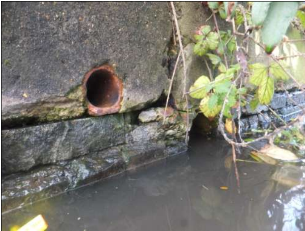
Photograph 41: Ch 250m – 2# open pipes
