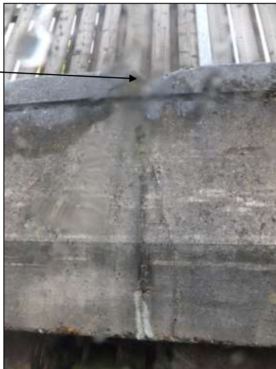
Photograph 14: Ch 114m – Open crack with spalled concrete adjacent to an outfall pipe.
