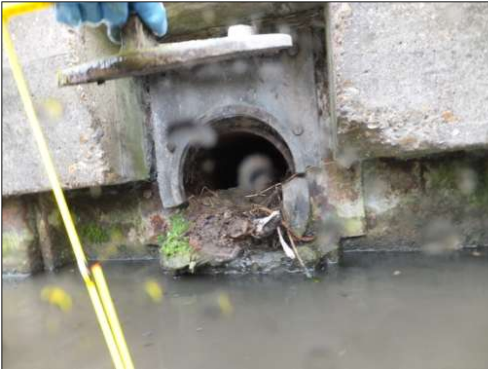
Photograph 29: Ch 190m – Outfall pipe blocked with debris..
