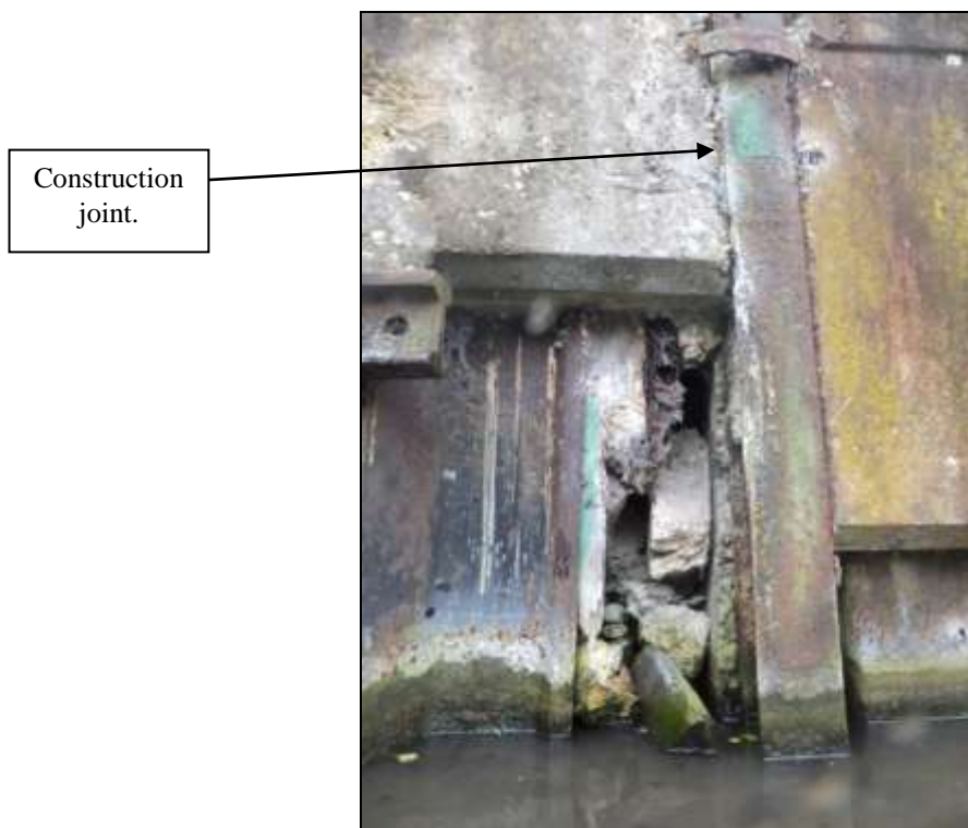
Photograph 6: Ch32 – Void back filled with loose rubble.
