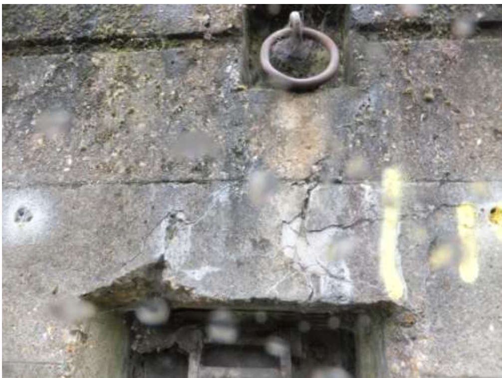
Photograph 30: Ch 210m – Defective area of concrete above capping beam.
