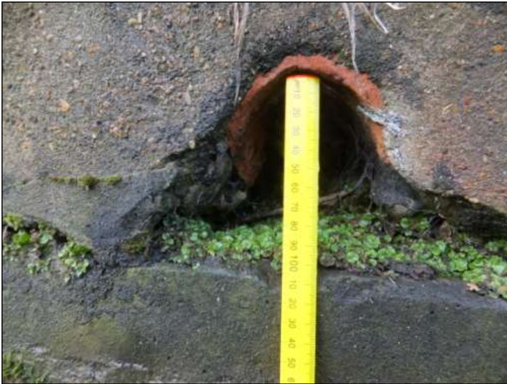
Photograph 38: Ch 240.5m – Open pipe.
