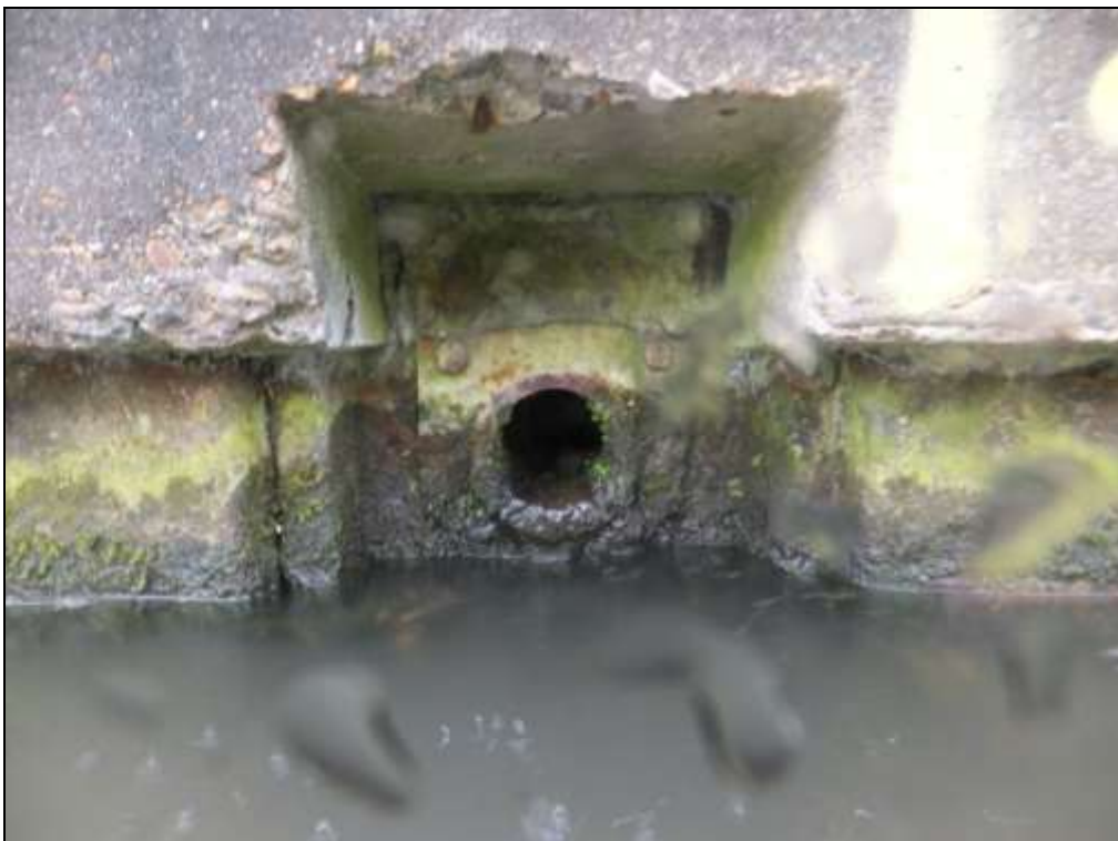
Photograph 32: Ch 230m – Outfall pipe with missing flap valve.
