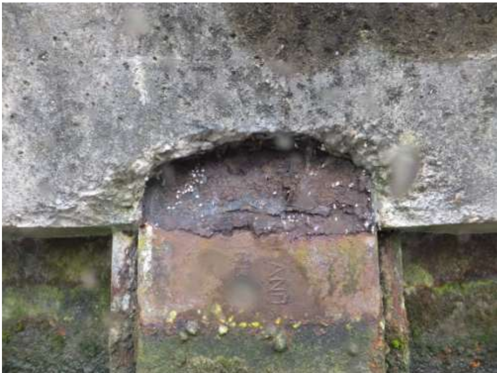
Photograph 18: Ch 86m – Spalling of the concrete capping beam as a result of steel de-lamination.
