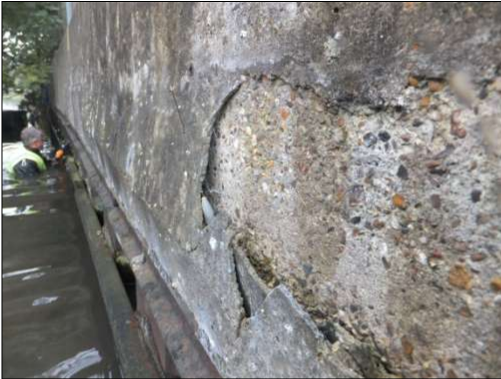
Photograph 5: Ch 16.5 – De-lamination of the render layer.
