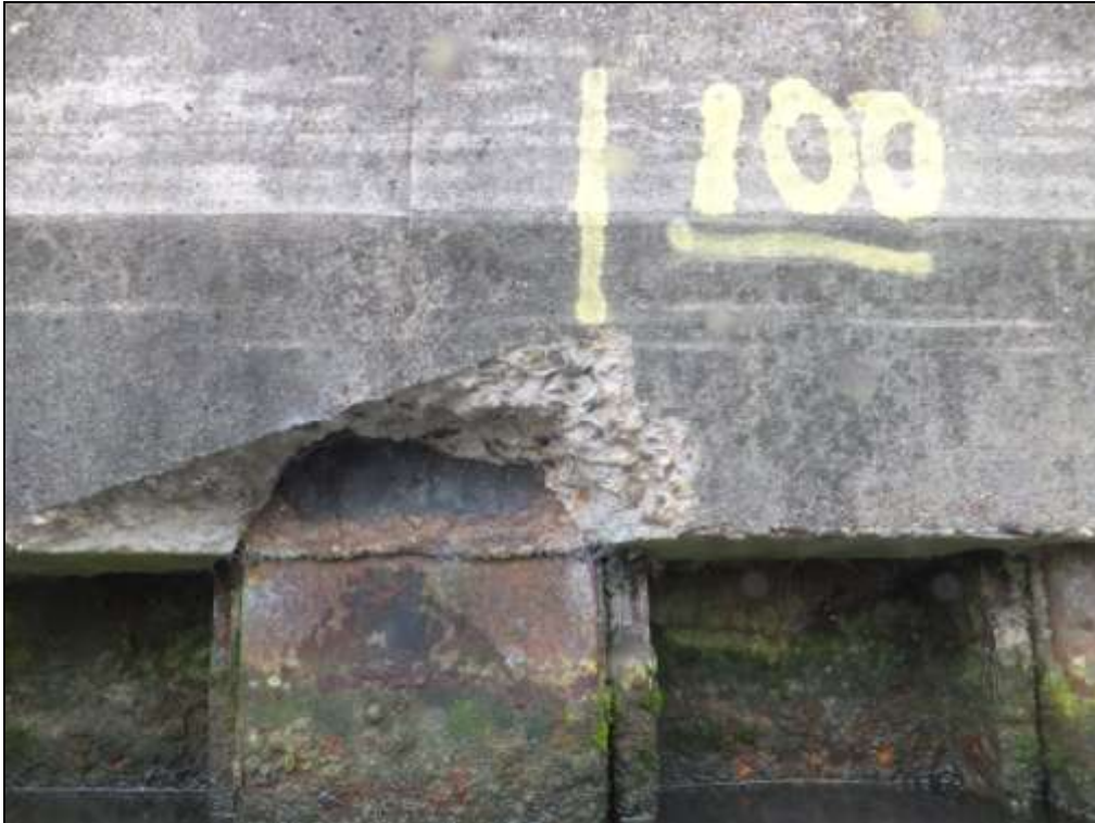
Photograph 19: Ch 100m – Spalling of the concrete capping beam, probably as a result of steel de-lamination.
