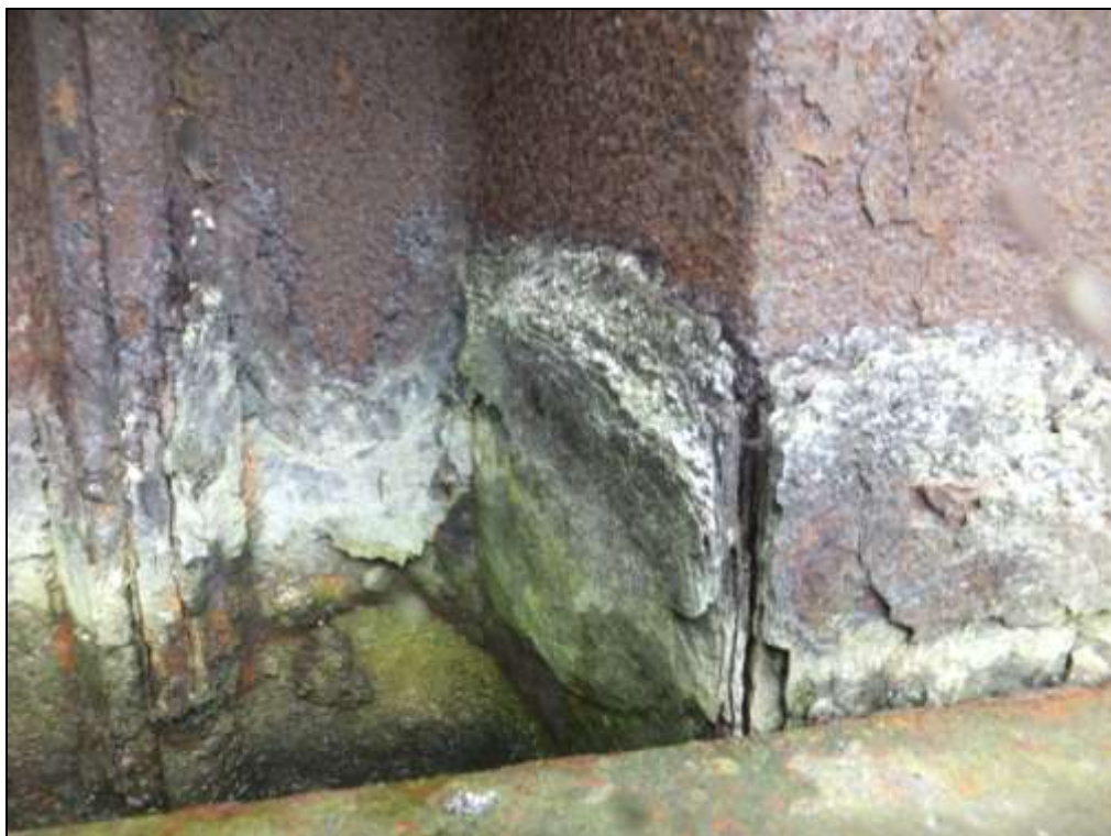
Photograph 4: Ch 0m – 9m – De-lamination of the steel in the splash zone.
