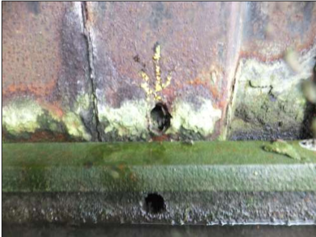
Photograph 3: Ch 1m – Hole in sheet pile wall.
