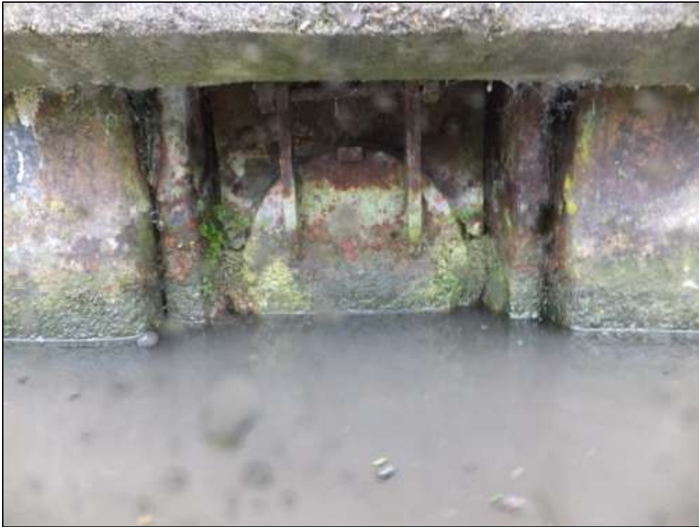
Photograph 17: Ch 70.5m – Outfall pipe fitted with a seized flap valve.
