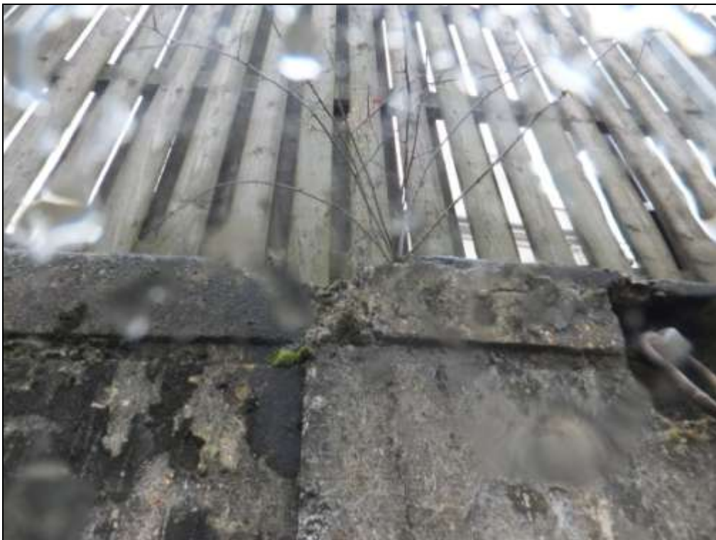
Photograph 26: Ch 162m – Vegetation causing spalling.
