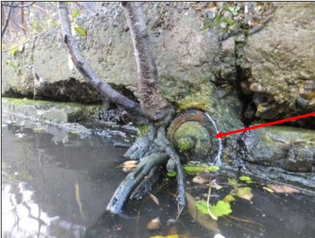
Photograph 35: Ch 265.5m – Vegetation and blanked pipe.
