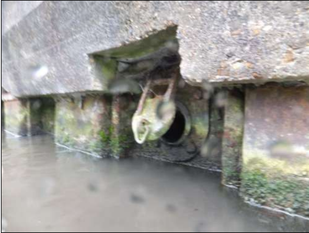
Photograph 31: Ch 196 – Outfall pipe fitted with a seized flap valve.
