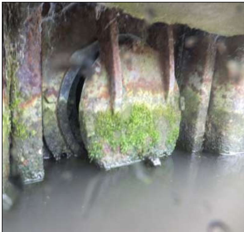
Photograph 12: Ch 11m – Outfall pipe fitted with a seized flap valve.
