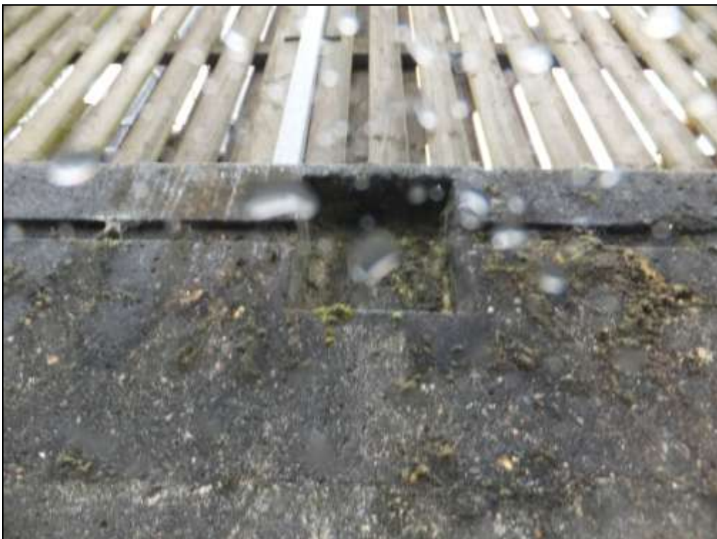
Photograph 10: Ch 176m – Missing mooring ring.
