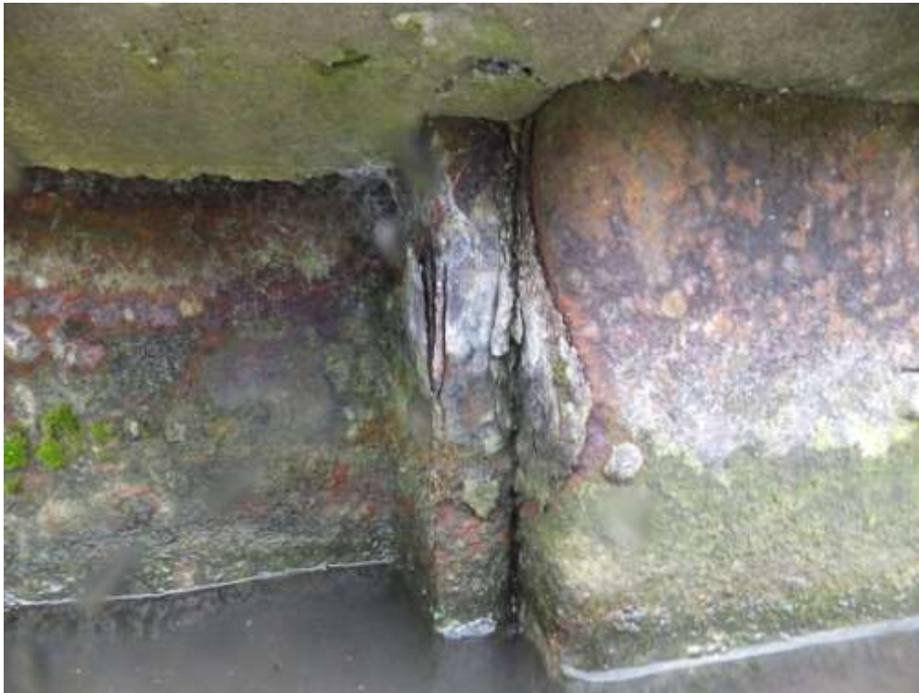
Photograph 16: Ch 30m – De-lamination of the steel adjacent to the pile clutch.
