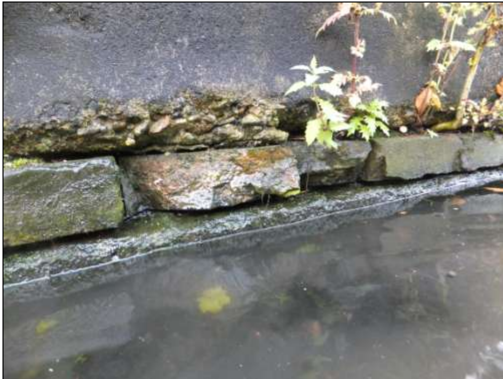
Photograph 37: Ch 260m – Missing mortar joints.
