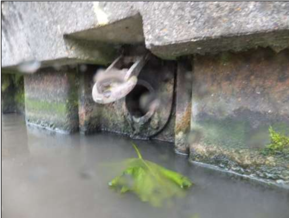
Photograph 27: Ch 175m – Outfall pipe fitted with a seized flap valve.
