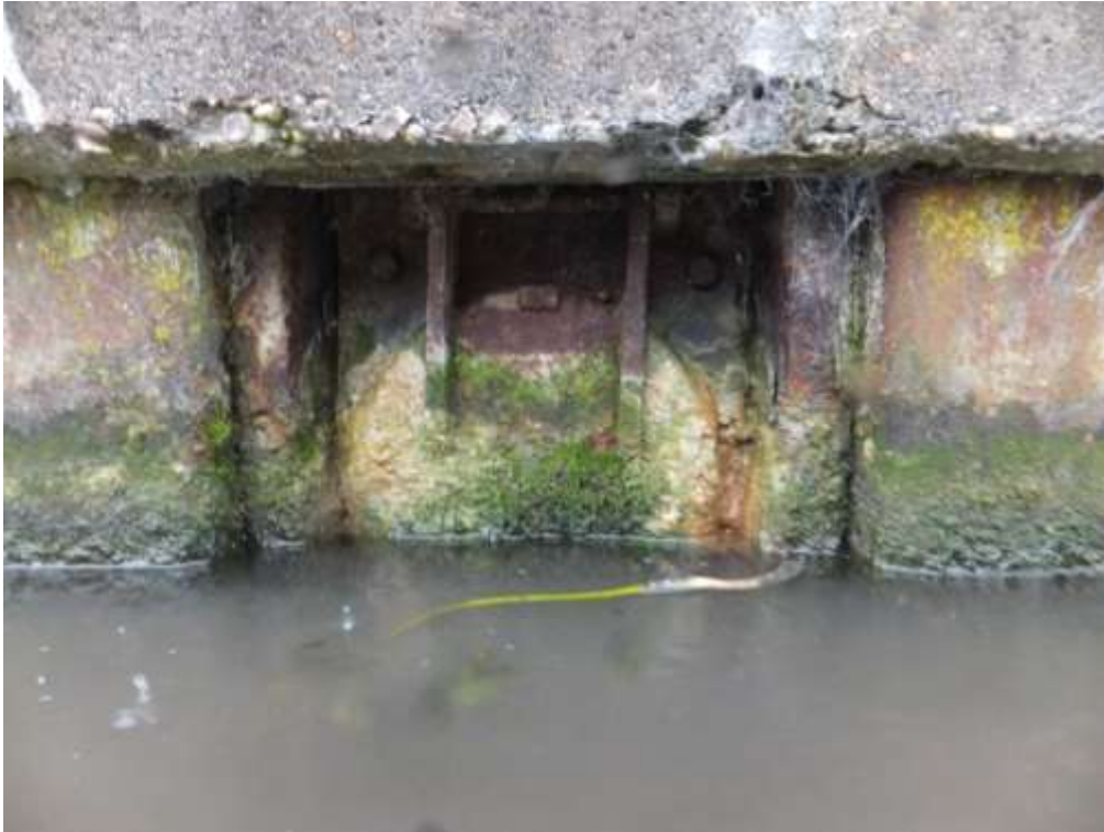
Photograph 21: Ch 98m – Outfall pipe fitted with a seized flap valve.
