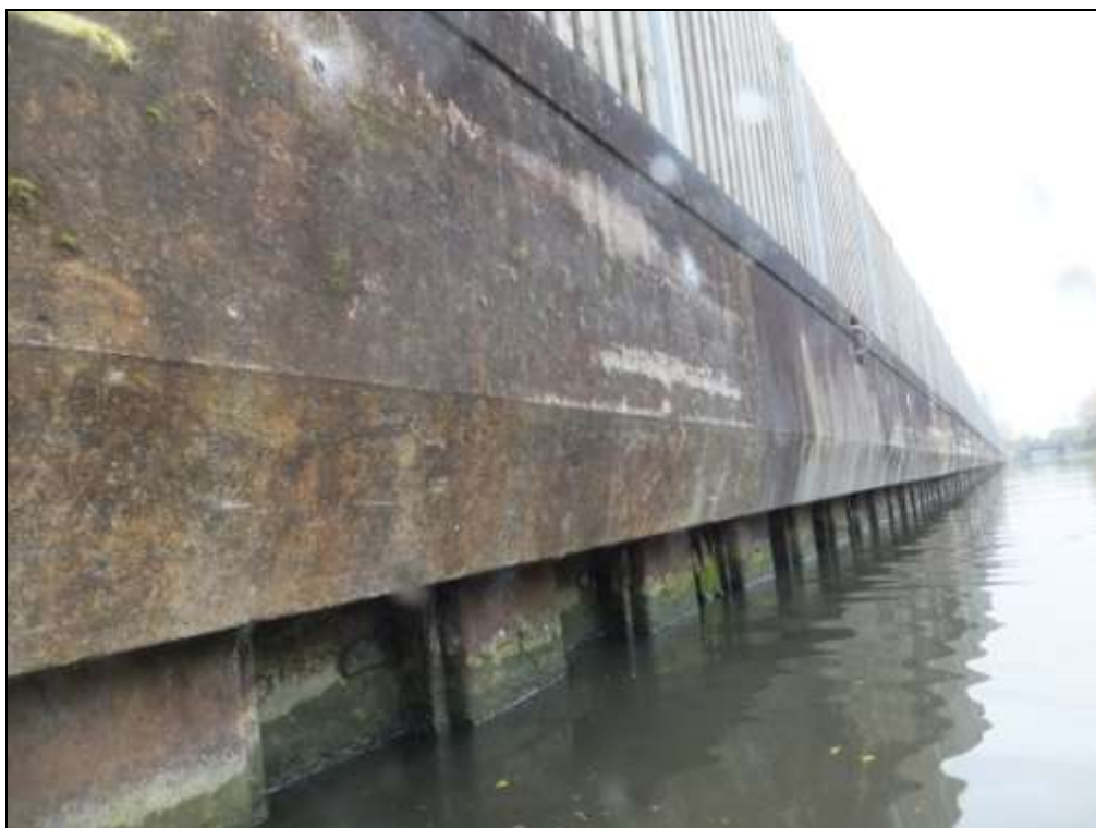
Photograph 8: Ch 9m – View of the canal retaining wall looking West along the structure.
