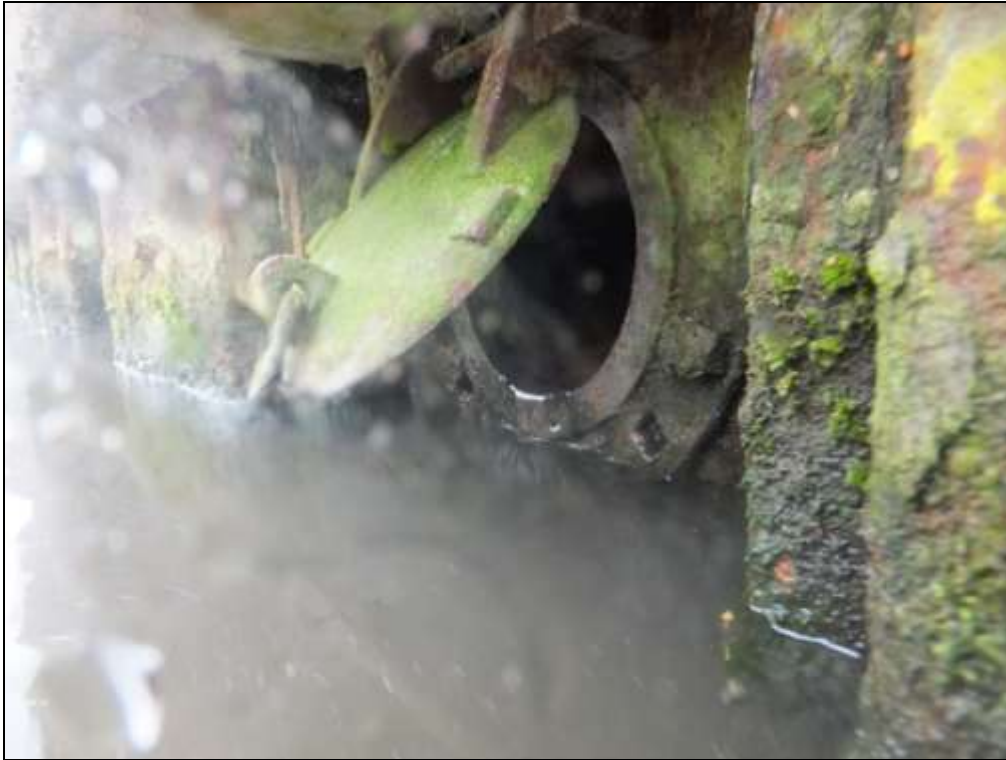
Photograph 23: Ch 114 – Outfall pipe fitted with a seized flap valve.
