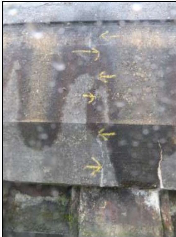
Photograph 13: Ch 56m – Hairline crack with efflorescence leaching at its base.
