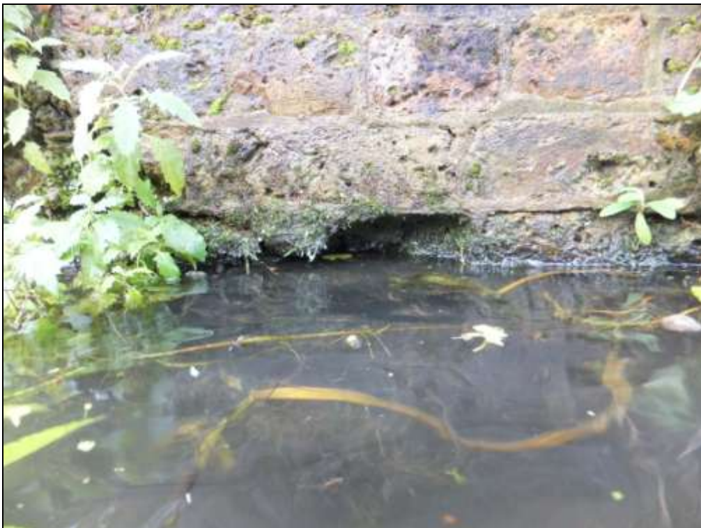
Photograph 36: Ch 235m Void in wall below the waterline.
