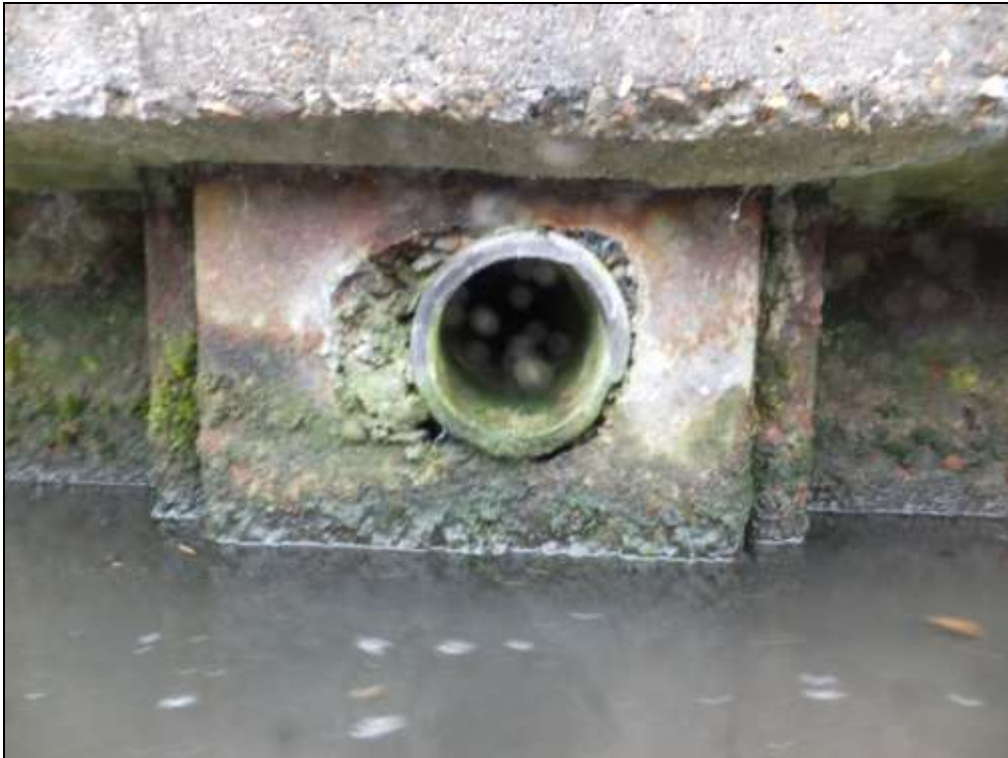
Photograph 25: Ch 159m – Open pipe.
