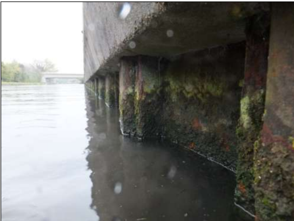
Photograph 22: Ch 113m – Misalignment of piles.
