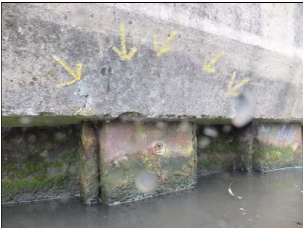
Photograph 20: Ch 95m – Cracking of the pile capping beam due to de-lamination of steel.
