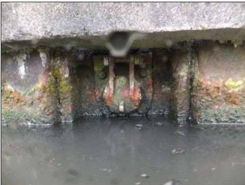
Photograph 24: Ch 136m – Outfall pipe fitted with a seized flap valve.
